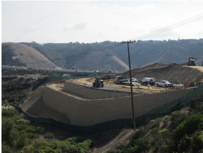
Photo 2: Construction activities associated with erecting the upper retaining wall to obtain final grade of the substation pad site continued during this reporting period.
