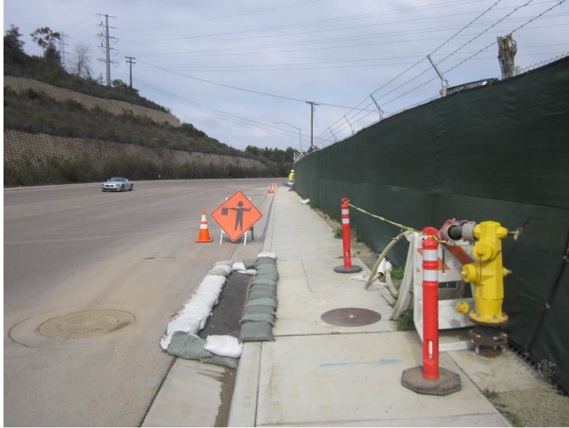
Photo 3: Traffic signage has been placed along Mira Sorrento Place notifying motorists of construction activities in accordance with MM-TT-1.
