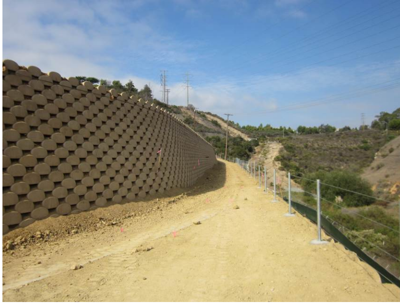
Photo 1: An access road has been constructed between the lower and upper retaining walls in order to provide access to a retention basin located in the southwest portion of the project site. A safety fence has also been constructed along the perimeter of the lower retaining wall.
