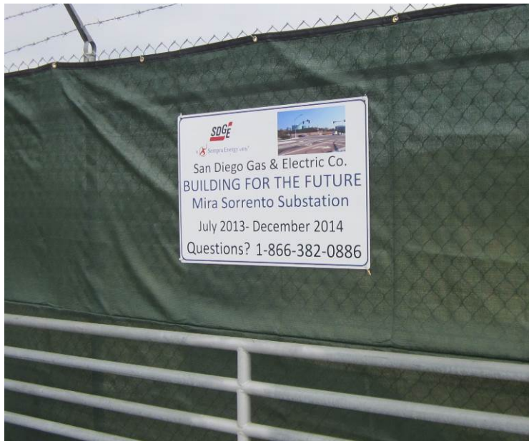
Photo 4: Signage has been placed at the intersection of Mira Sorrento Place and Vista Sorrento Parkway notifying the public of the construction activities. A toll-free number has been established by SDG&E for responding to any questions or complaints in accordance with MM-NOI-2.
