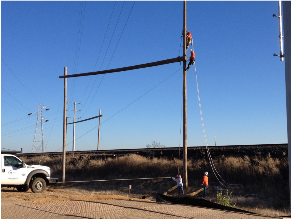
Figure 1: Wood pole guard structure.
