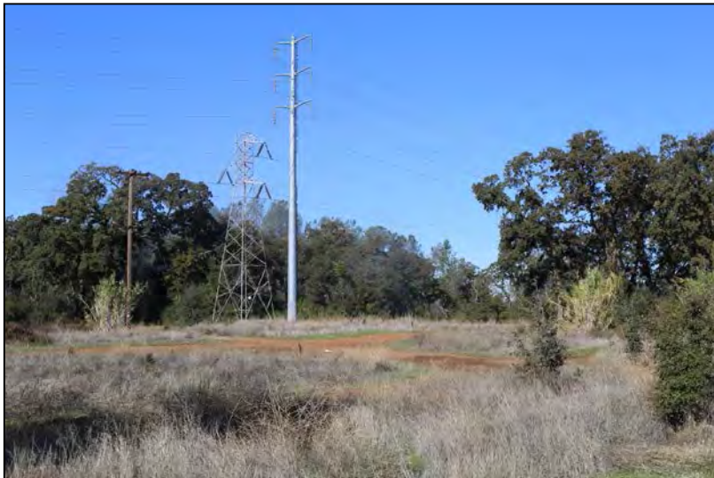
Photograph 3 - View of South of Palermo Single-Circuit Line and adjacent power line from North Villa Avenue (Palermo)
