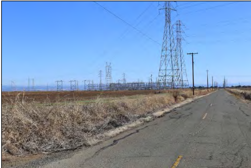
Photograph 25 - View of Rio Oso Single-Circuit Sub-Line Segment Loop, adjacent power line, and Rio Oso Substation from Hicks Road
