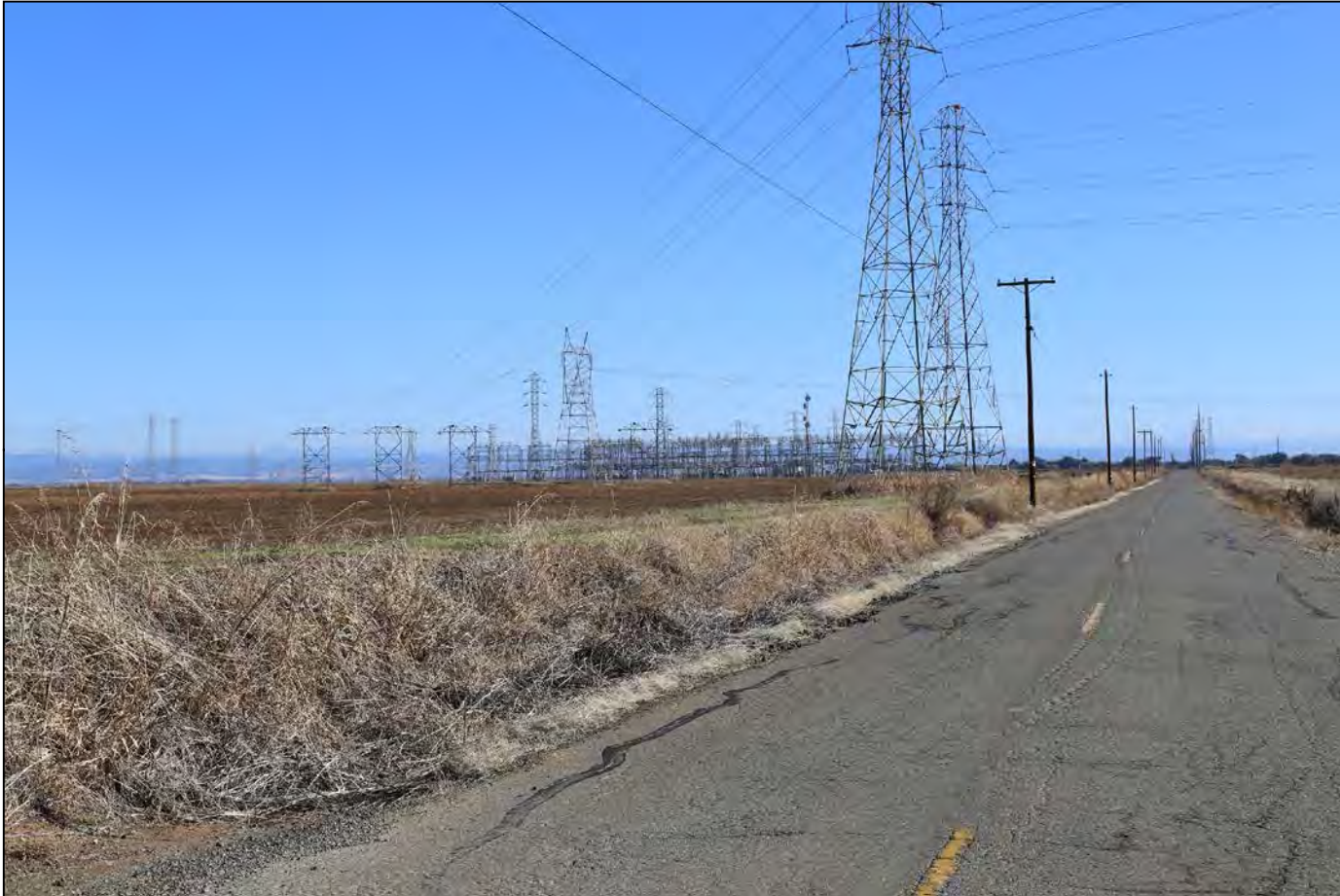
Existing view of the Rio Oso Single-Circuit Sub-Line Loop and Rio Oso Substation from Hicks Road
