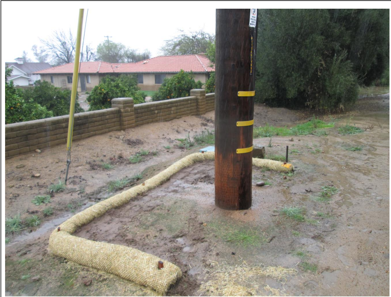
Photo 8: A Straw Wattle was observed installed around a pole replacement location in accordance with the SWPPP.
