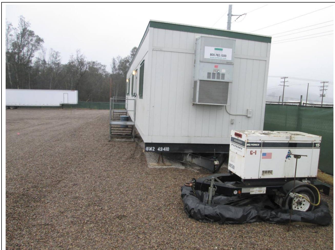
Photo 5: Temporary equipment at the Warnock Staging Yard (such as generators, above) were observed staged on visqueen for secondary containment in accordance with MM HYD-2.
