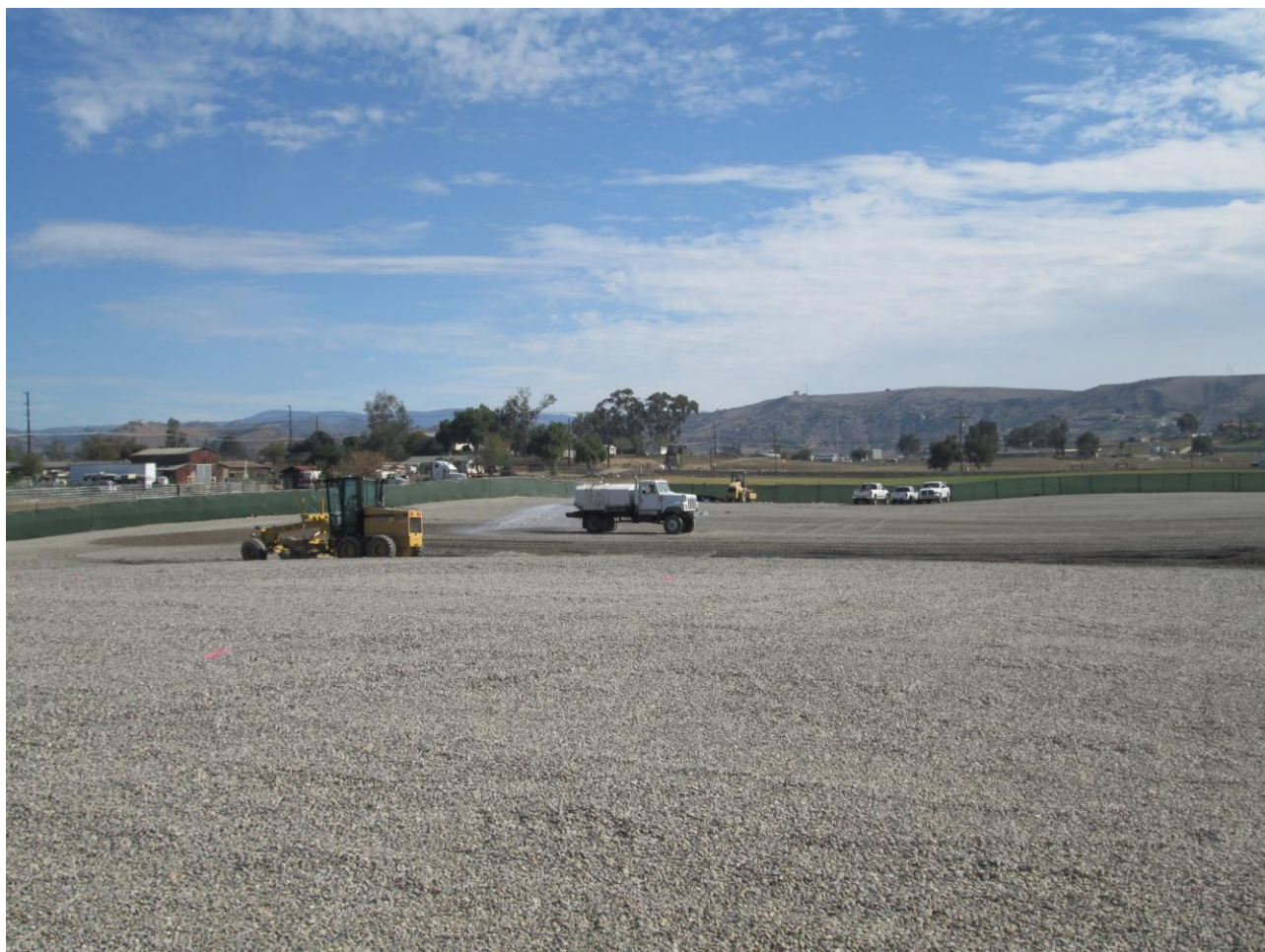
Photo 4: Water trucks were observed at the Warnock Staging Yard applying water prior to grading activities and during gravel spread to prevent fugitive dust in accordance with APM BIO-1.
