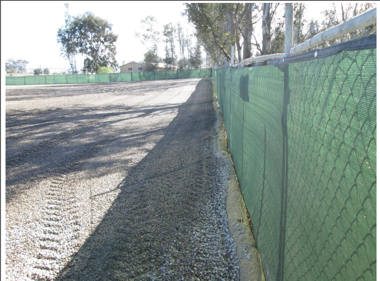
Photo 1: Opaque mesh screening material has been placed along the perimeter chain-link fence at the Warnock Staging Yard in accordance with APM AES-1.
