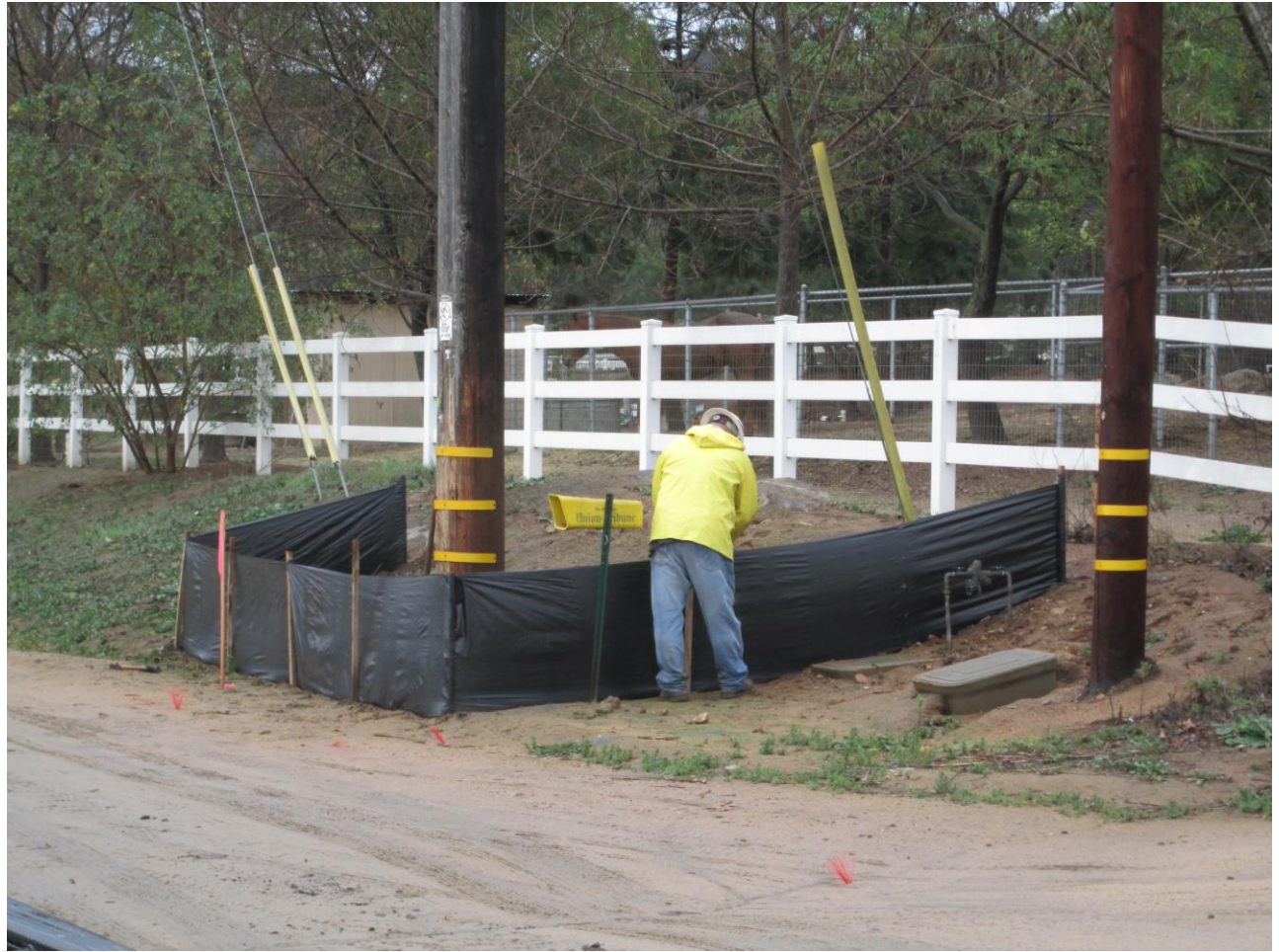
Photo7: Silt Fence was observed being installed around pole locations in accordance with the SWPPP.
