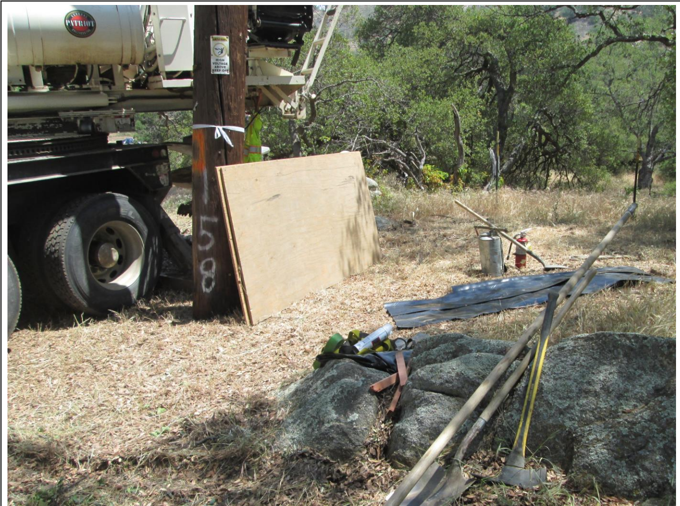
Photo 2: During air track drilling activities, fire tools were staged on site in accordance with APM HAZ-2 and the Project Fire Plan. Environmentally Sensitive Areas were delineated with metal T-posts for avoidance in accordance with MM CUL-1.
