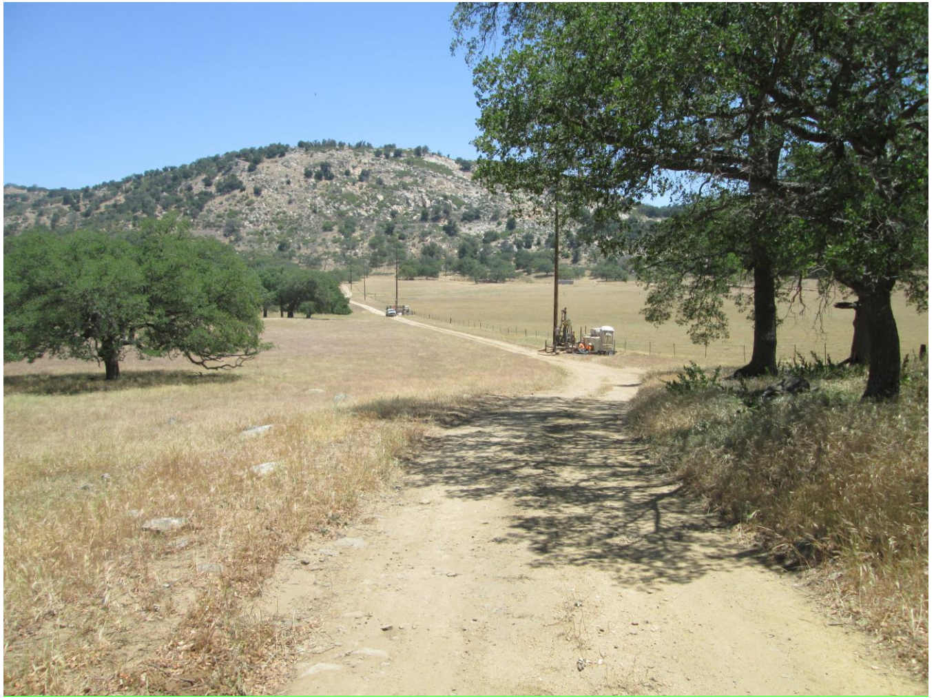
Photo 1: Micropile construction crews were observed drilling micropiles (pictured), and strength testing micropile foundations during the reporting period.
