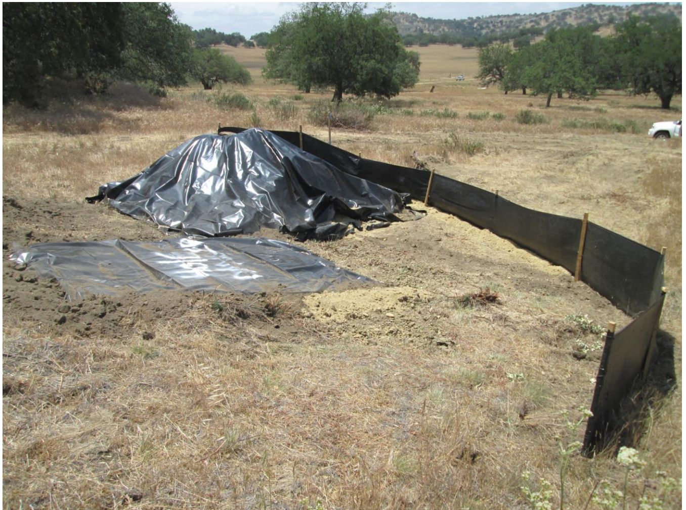
Photo 6: Sediment control BMPs implemented along the project alignment included the use of silt fencing and the covering of dirt stockpiles in accordance with the Project SWPPP and APM-HYD-1. Previously drilled pole holes were observed covered to prevent potential wildlife entrapment in accordance with MM-BIO-3.
