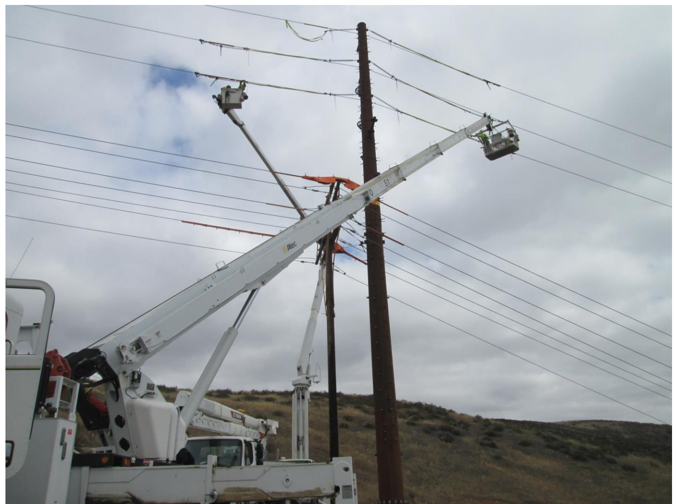
Photo 4: Construction crews were observed adjusting conductor line sag and clipping-in conductor lines.
