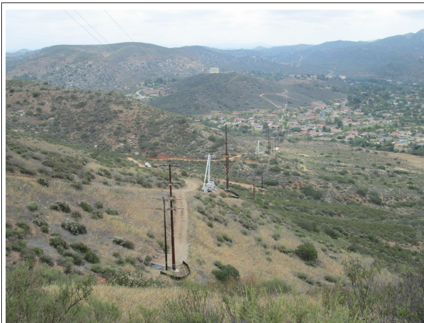
Photo 3: Wire stringing activities were observed during the reporting period, and water tenders were observed within 2 minutes travel time of work locations in accordance with APM-HAZ-2 and the Project Fire Plan.
