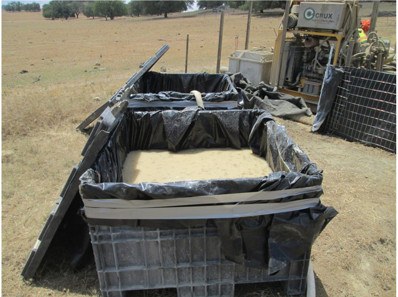
Photo 7: In accordance with the Project SWPPP and APM-HYD-1, groundwater encountered during micropile foundation hole drilling was contained with silt fencing, and transferred into containment boxes (pictured) that were emptied into a retention basin at the Santa Ysabel Staging Yard.
