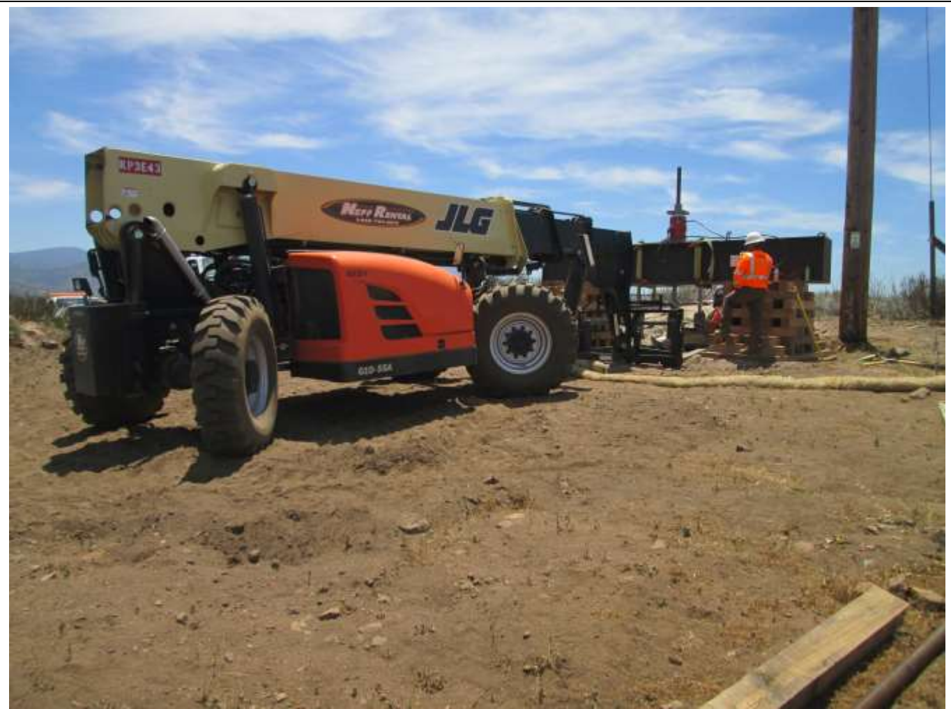
Photo 2: Micropile foundation strength testing was observed during the reporting period, which involves the use of a wooden cribbing, a steel beam, and a forklift.
