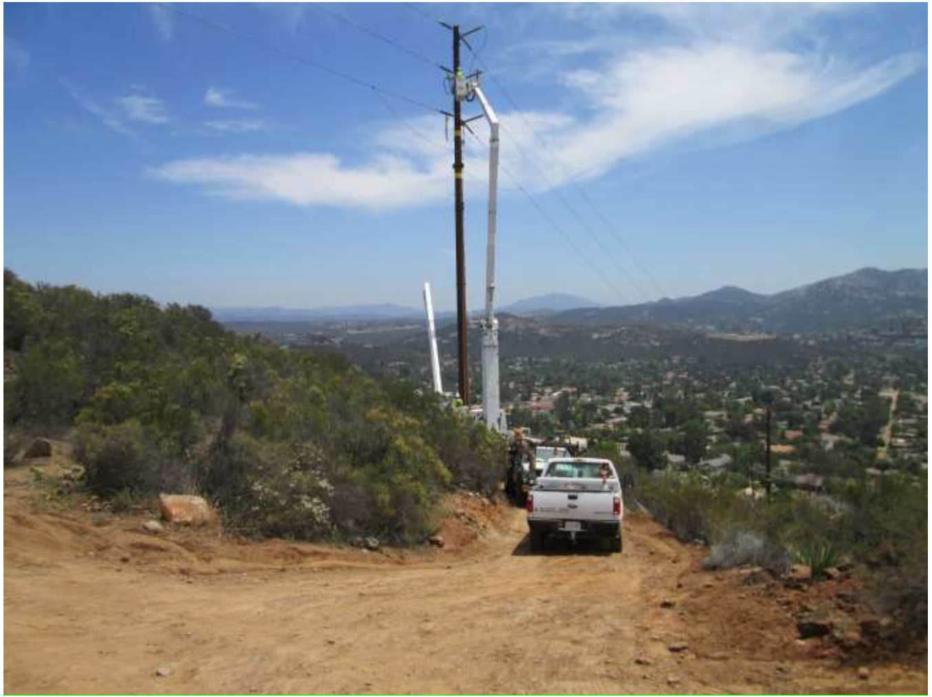
Photo 1: Construction crews were observed conducting wire stringing activities, which included dead-ending and sagging the wire (pictured above).
