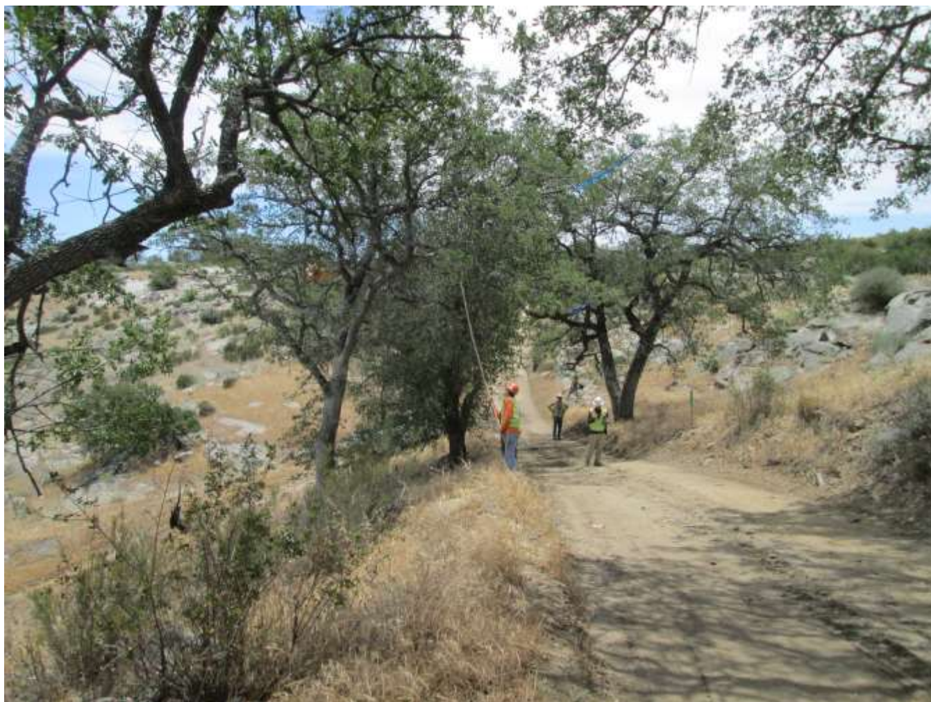
Photo 3: In accordance with APM BIO-1, MM BIO-2, and MM BIO-4, a tree trimming crew, with direction from the on-site biological monitor, was observed using a hand saw for tree trimming activities to limit noise that could potentially disturb to an active bird's nest located just off the access road.
