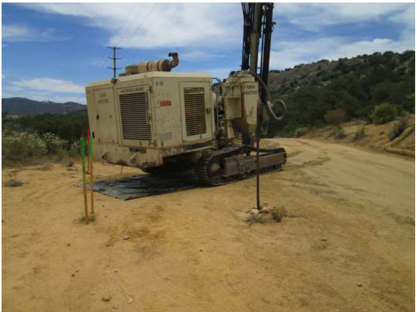
Photo 5: Sensitive plant species were marked for avoidance with green colored stakes in accordance with APM BIO-1, and visqueen was observed being used beneath staged equipment to prevent potential leaks/spills from being discharged into the soil in accordance with MM HYD-2.
