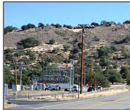
Santa Ysabel Substation
