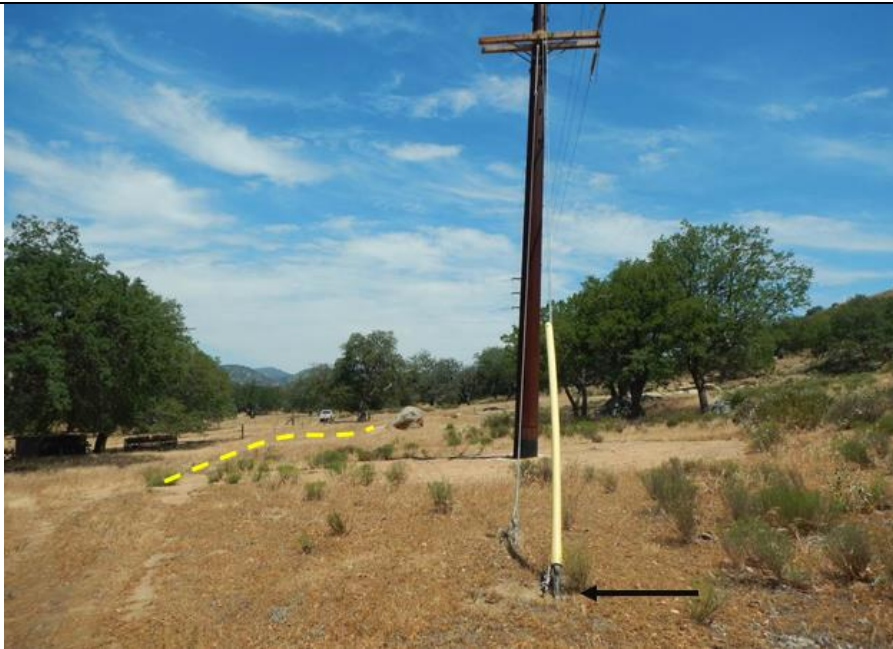
Photograph 6: View of existing pole (151(B)) that requires modifications including location of guy anchor removal (black arrow), and existing access road (yellow) to pole, facing north.
