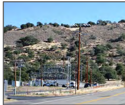
Santa Ysabel Substation
