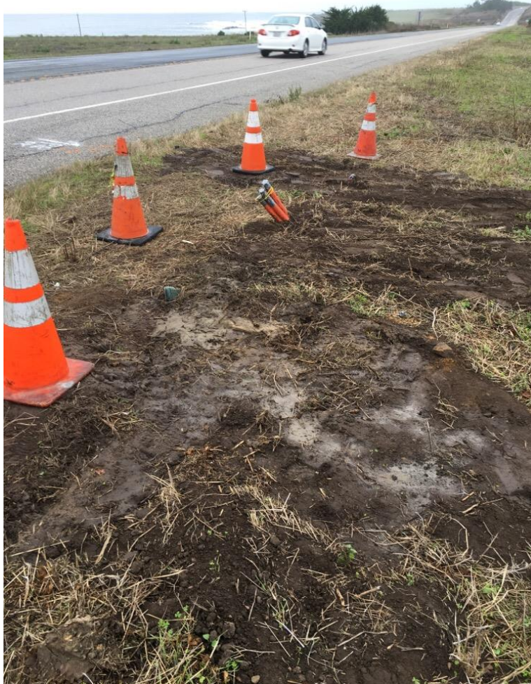
Photo 6: HDD installation area.
