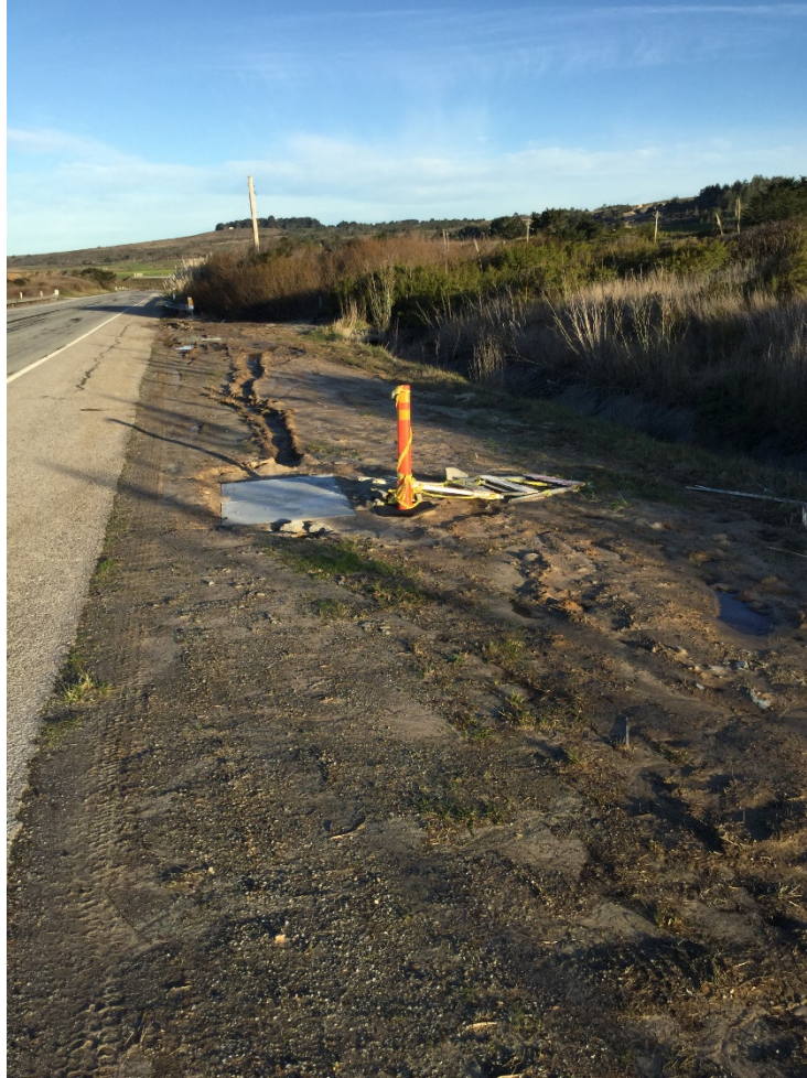
Photo 3: Tire ruts on Highway 1 northbound shoulder, mile marker 5.38. Barricade, cone, and flagging remain on site.
