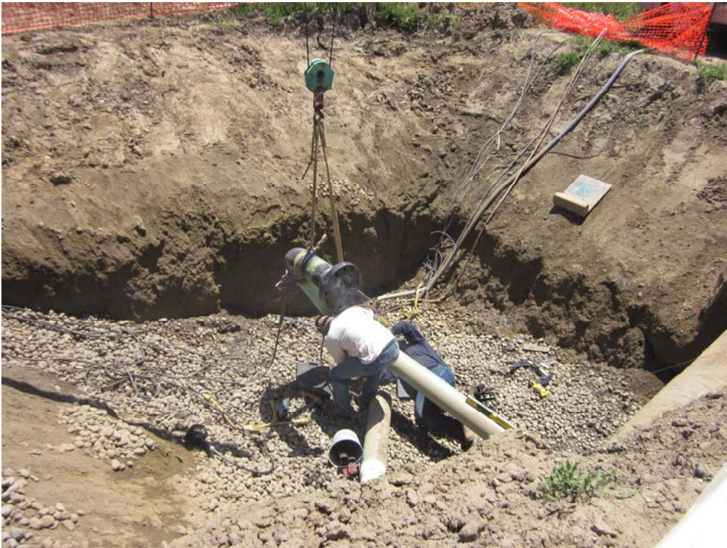
Photo 2: PG&E gas line 172 connection at the remote well pad site.
