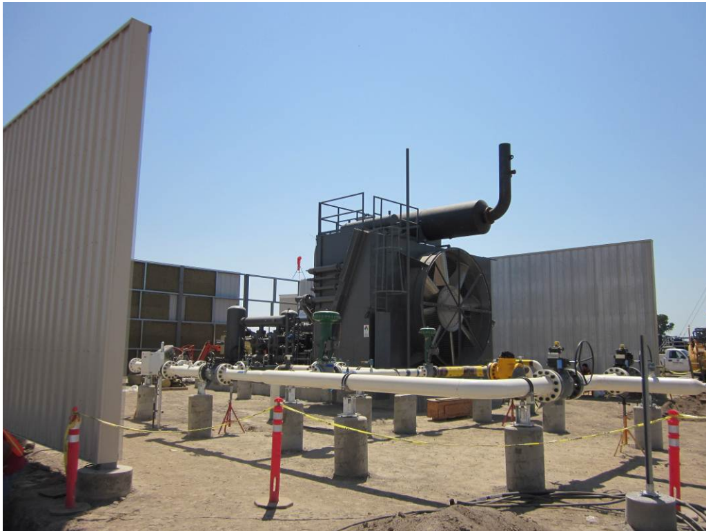
Photo 2: Soundwall work at temporary compressor placed at the remote well pad site.
