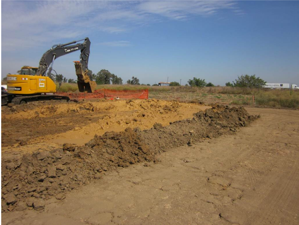
Photo 3: HDD at Interstate 5. Drill mud being contained and loaded into trucks for hauling offsite and treatment.
