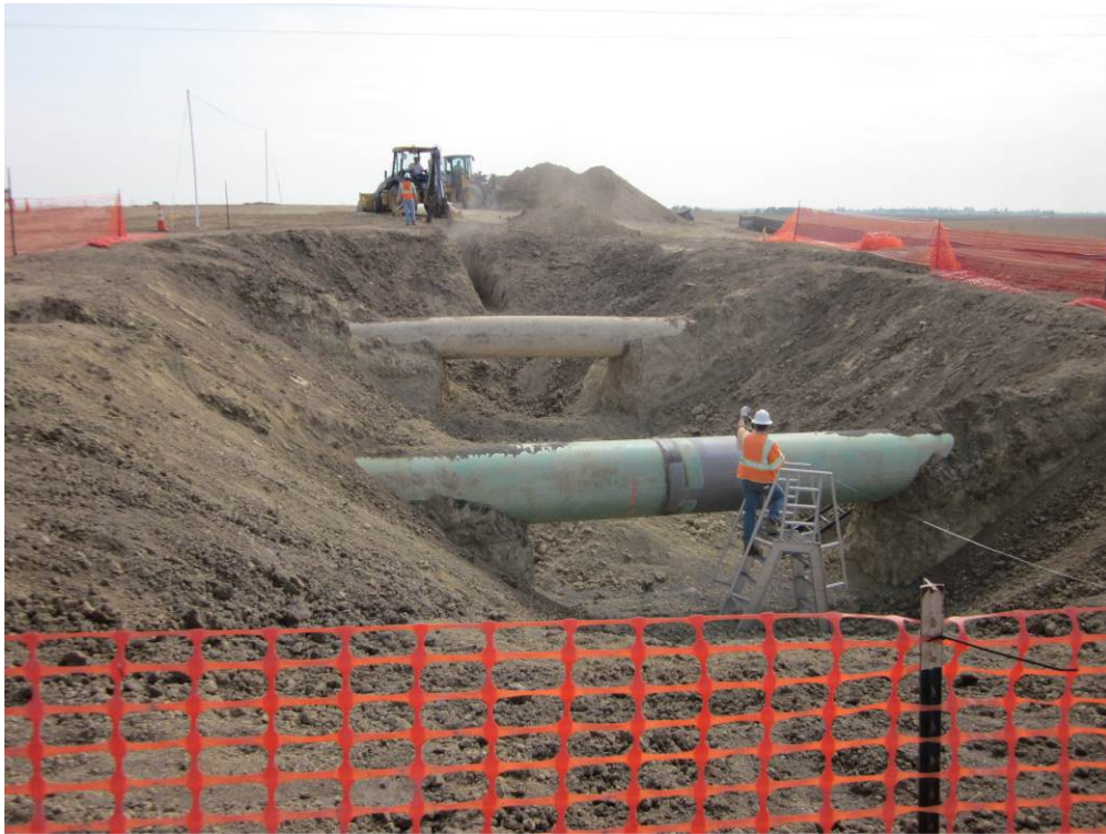
Photo 6: PG&E crew working at the 400/401 Line Interconnect. The 400 and 401 lines have been excavated and trenching is underway for the connection to the Metering Station.
