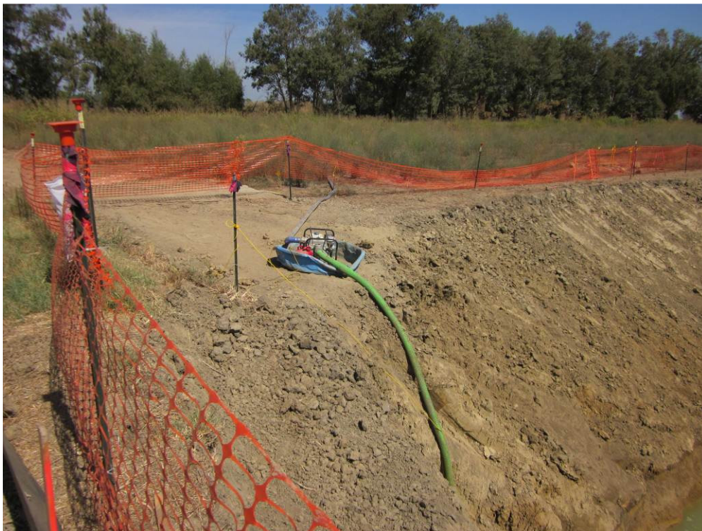
Photo 4: Dewatering operations at the D-24 auger bore onto non-approved parcel. Dewatering at this location has ceased pending submittal of the revised Dewatering and Discharge Plan.
