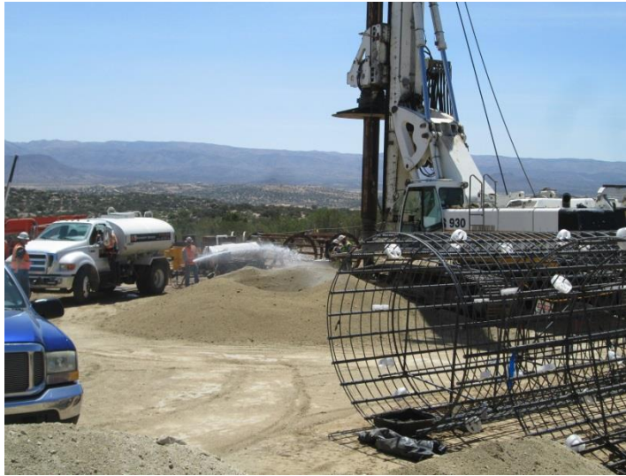
Photo 3: Water trucks were observed being utilized during foundation drilling in accordance with MM-BIO-4a and the Dust Control Plan.
