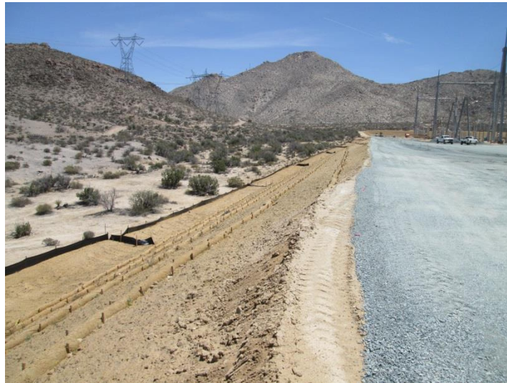
Photo 6: BMP's consisting of straw wattles, silt fence and soil stabilizer have been put in place along slopes of the ECO Substation to minimize erosion in accordance with MM-HYD-1 and the SWPPP.
