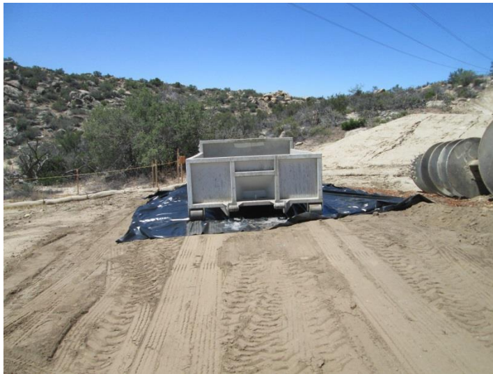
Photo 4: In accordance with MM-HYD-1 and the SWPPP, concrete washouts are utilized during concrete pours associated with steel pole foundations.
