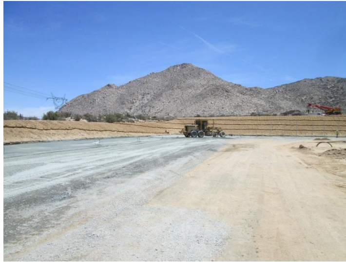
Photo 5: Class II fill being placed within the approved work limits at the ECO Substation.
