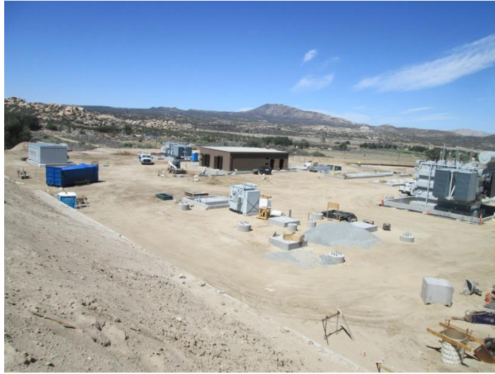
Photo 7: The control shelter at the Boulevard Rebuild Substation has been treated with an Otay Ranch Brown color tone in accordance with the Surface Treatment Plan and MM-VIS-3g.
