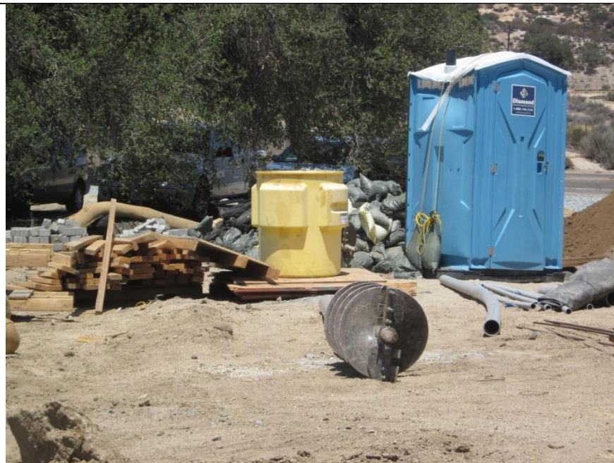
Photo 6: Spill kit observed on site in the case of a hazardous materials spill in compliance with MM HAZ-1a.
