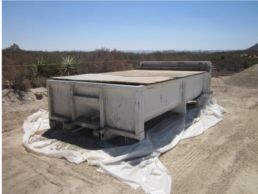
Photo 1: A concrete washout basin was observed in good condition along the ROW.
