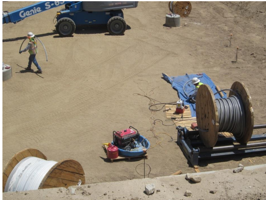
Photo 5: Staged generators and equipment were equipped with drip pan containment in compliance with MM HAZ-1a.
