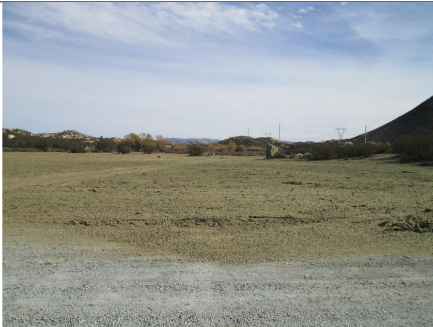
Photo 2: Restoration activities were observed being completed at the Lake Domingo Construction Yard during this reporting period. Crews were observed decompacting soils prior to applying a seed mix in accordance with MM-BIO-1D and the Habitat Restoration Plan.
