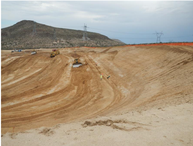
Photo 3: Construction activities associated with rough grading of the 500 kV substation pad at the ECO substation site continued during the week of September 2.
