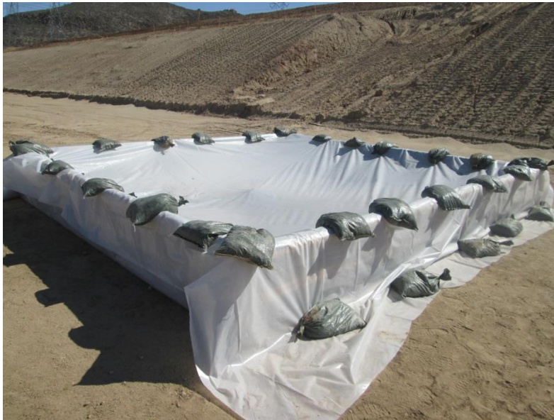
Photo 4: A concrete washout basin is established in preparation of pouring concrete foundations at the 138/230 kV pad site in accordance with the SWPPP and MM-HYD-1.
