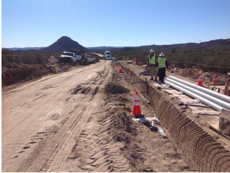
Photo 1: Archaeological and Native American monitors were observed monitoring construction activities along the 138kV underground transmission line in accordance with CUL-1D.
