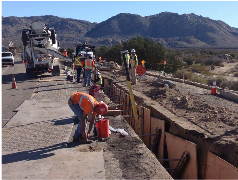
Photo 3: Traffic signage and steel plates were observed in place in areas of inactive construction in accordance with the MM TRA-1.
