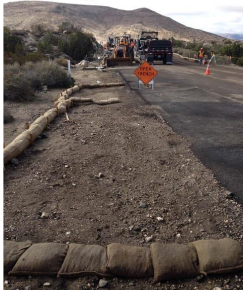
Photo 4: Erosion control devices consisting of gravel bags and straw wattles were observed installed and secured along Old Highway 80 in accordance with MM HYD-1.
