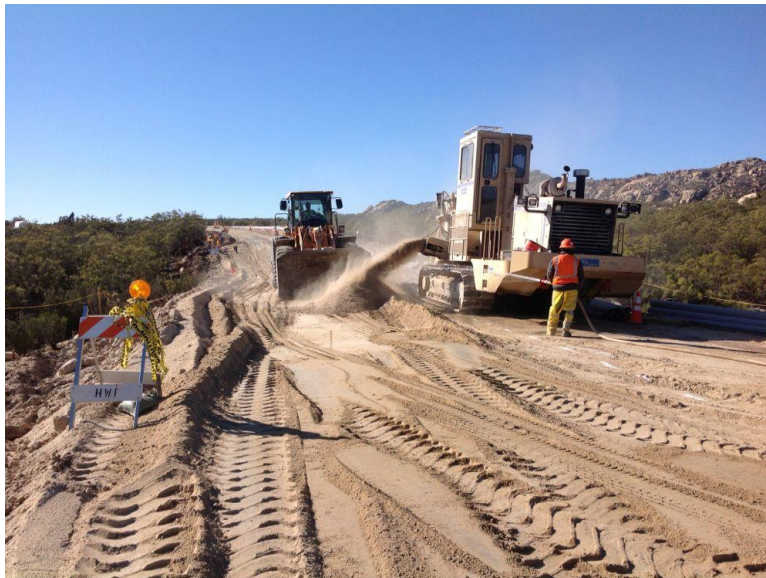
Photo 2: Water was observed being utilized during excavations to minimize fugitive dust emissions in accordance with MM AQ-1 and MM BIO-4a.
