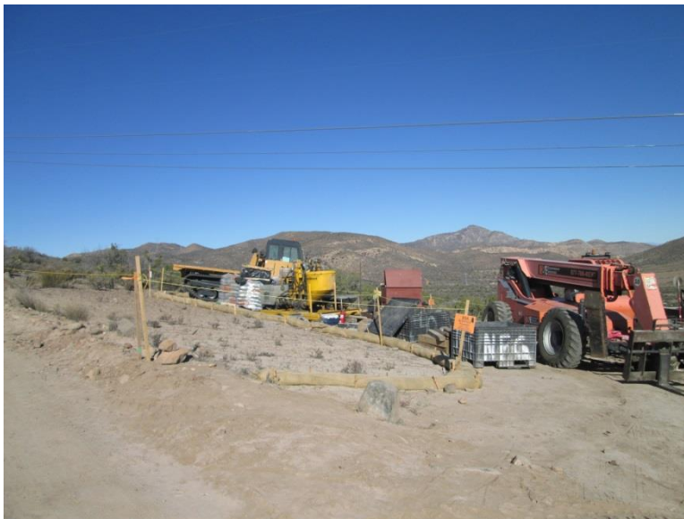
Photo 8: ESAs were observed flagged for avoidance during micro pile construction at SP- 76 in accordance with MM-CUL-1D.
