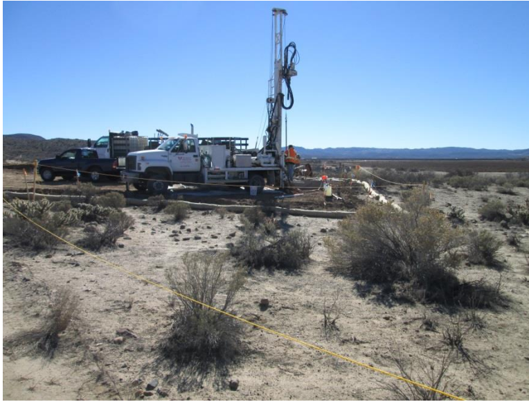
Photo 7: Archaeological monitors were observed present during geotechnical activities in accordance with MM CUL-1D. The drill rig shown above is staged over heavy plastic and straw wattles are in place to prevent potential leaks from being discharged into the soil.
