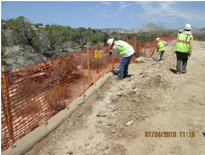
Photo 4: Construction crews were observed maintaining BMP's in good working order in accordance with MM-HYD-1.
