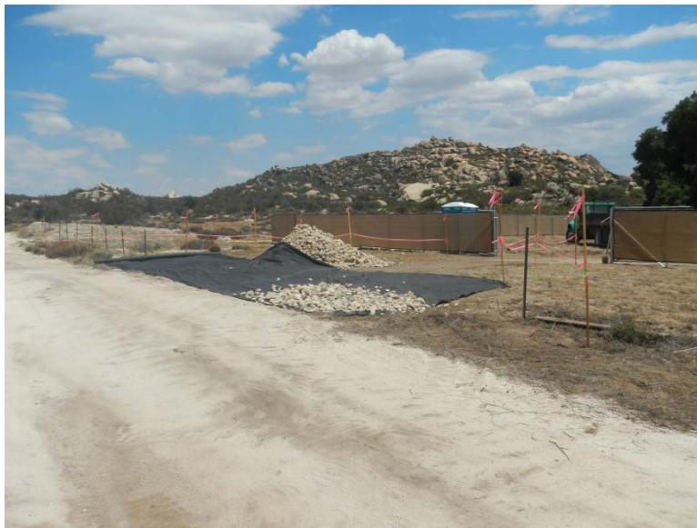
Photo 6: A rock apron has been constructed at the point of ingress/egress to the Jewel Valley Construction Yard to minimize trac-out along Jewel Valley Road in accordance with MM-BIO-4A and the Dust Control Plan.
