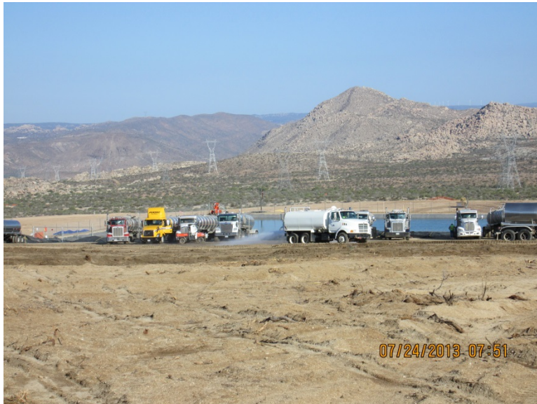
Photo 2: A temporary water retention pond has been constructed at the ECO Substation site for storage of construction water in accordance with Minor Project Refinement Request #001 (see Attachment C).
