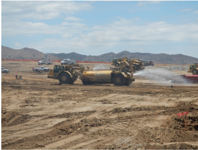
Photo 3: Water was observed being applied by the construction contractor for dust control and compaction purposes during earthwork activities in accordance with MM-AQ-1.
