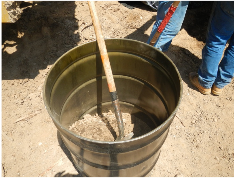
Photo 5: Construction crews remove stained soil in accordance with MM-HAZ-5a and the Spill Prevention Control and Countermeasure Plan.
