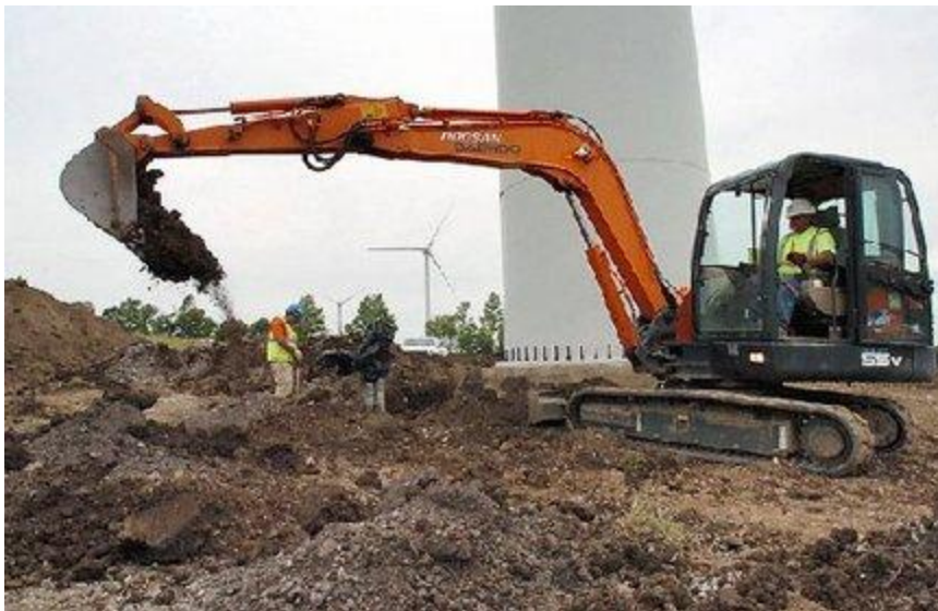
Michelle Gabel/The Post-Standard Scott Preston (right) and David Bajgerowicz, both of Fuller Excavating, clear away dirt near the foundation of a wind turbine in Fenner. Workers are reinforcing the foundations following the collapse of one of 20 wind turbines at the Fenner Wind Farm.
