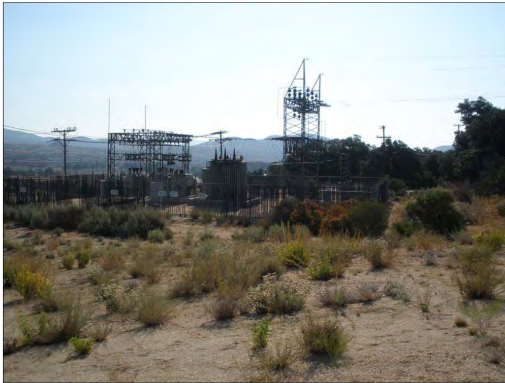
FIGURE 5-49. EXISTING BOULEVARD SUBSTATION VIEW EAST
