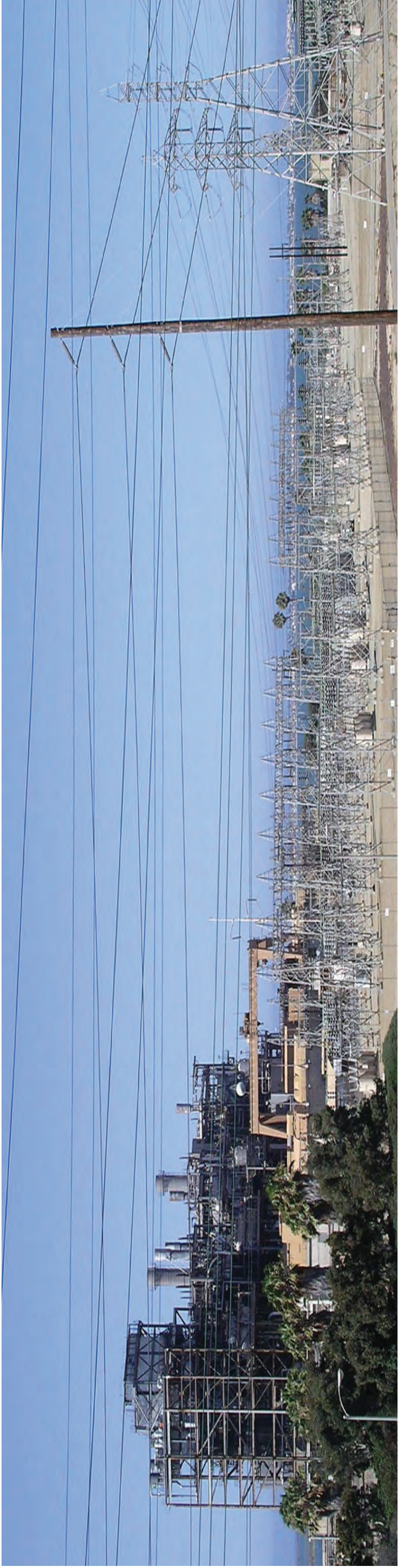
Existing Condition (View of the existing South Bay Substation and South Bay Power Plant, looking west from the L Street overpass)
