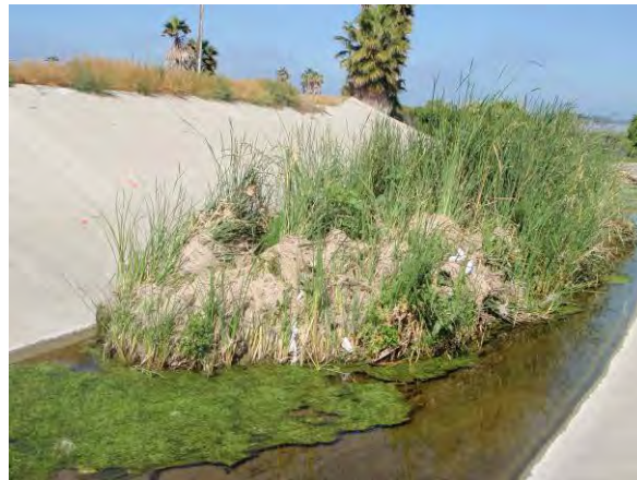
Telegraph Creek depicting vegetation blockage on accumulated.
