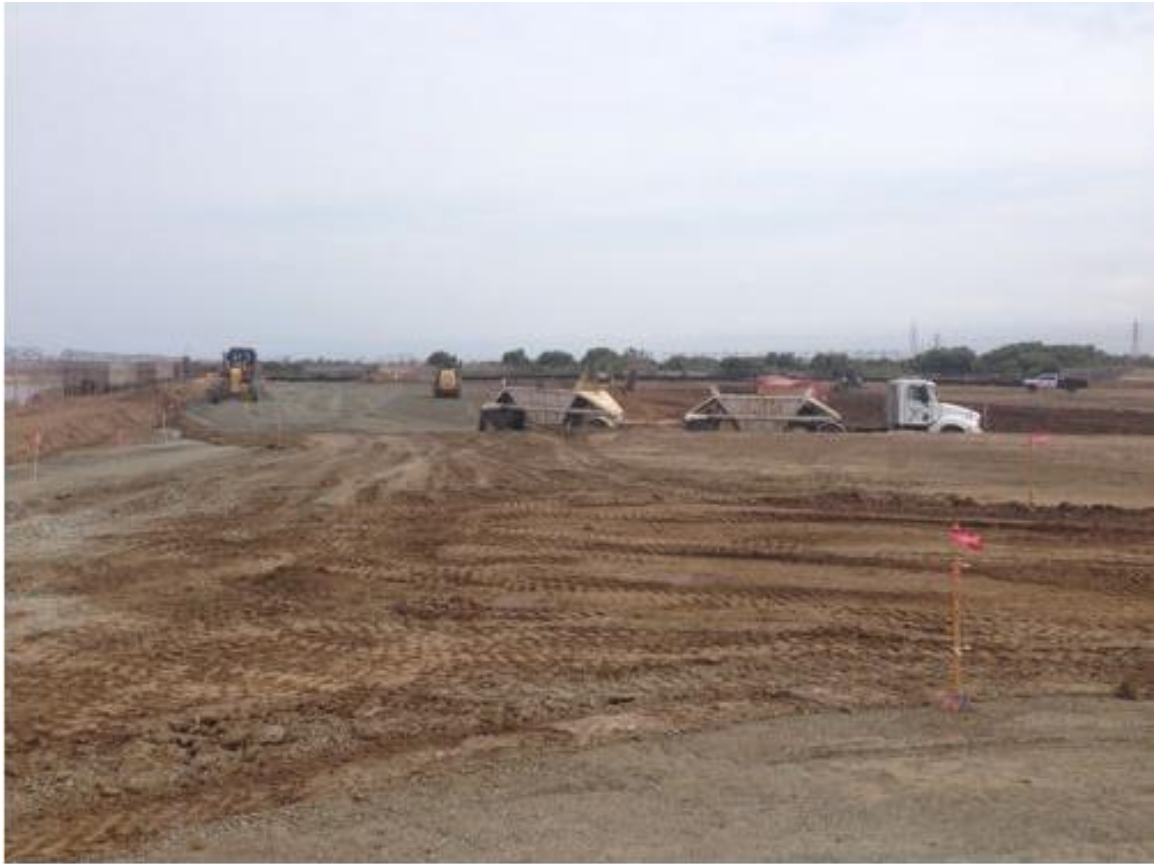
Photo 2: Import of fill material was observed at the Bay Boulevard Substation Site.
