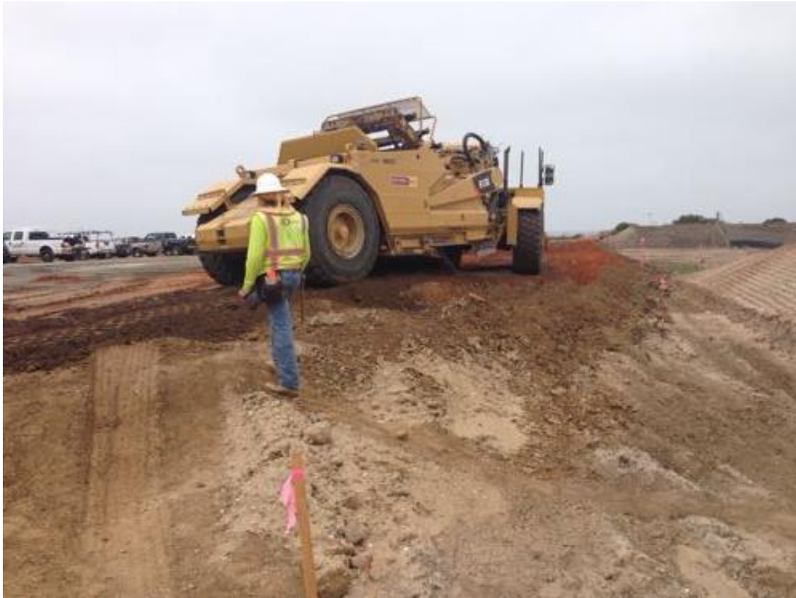
Photo 1: Rough grading and compaction of fill material was observed at the Bay Boulevard Substation Site.
