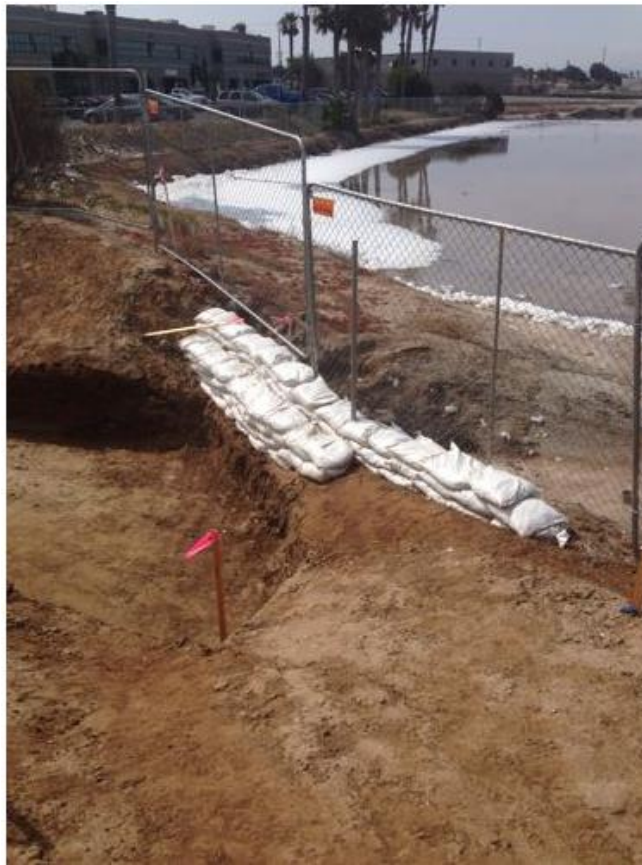
Photo 4: The gravel bag berm at the southwest corner of the project site, installed in accordance with the SWPPP, was observed intact, as well as other BMPs.
