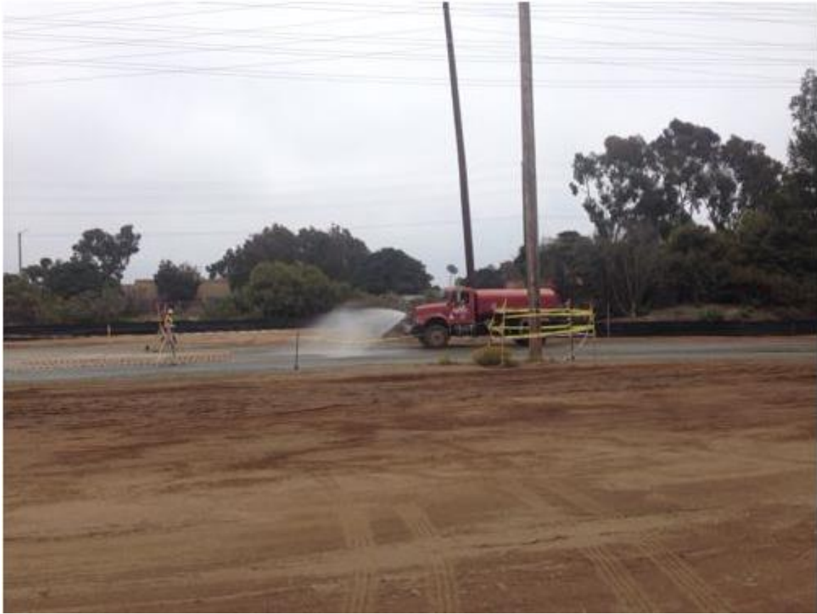
Photo 3: Water trucks were observed wetting roads and areas of active construction in order to prevent fugitive dust in accordance with APM-AIR-01.
