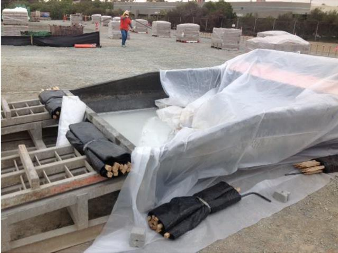
Photo 4: Designated concrete washout areas were available, covered, and marked on site in accordance with the SWPPP.
