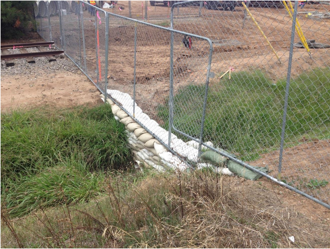
Photo 5: Gravel bags were installed at the southern entrance along the temporary perimeter fence to prevent off-site sediment discharge in accordance with the SWPPP.
