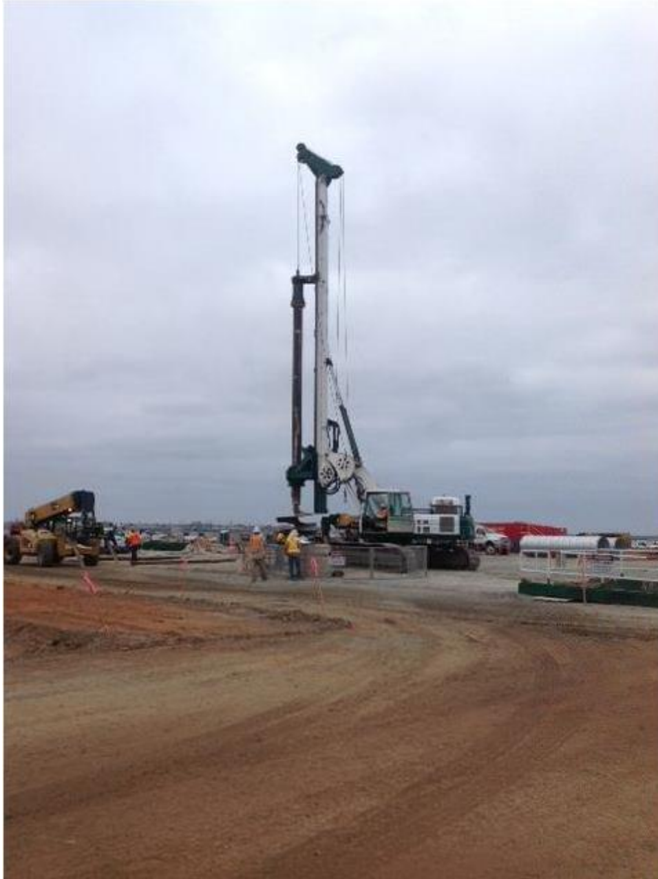
Photo 1: Drilling for tower foundations at the Bay Boulevard Substation. Monitors were observed on site during initial disturbance in accordance with MM-CUL-01 and APM-CUL-05, as applicable.
