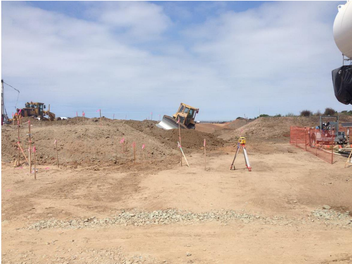
Photo 2: Placement of fill material north of the 230kV yard. No dust was observed during activities in accordance with APM-AIR-01.
