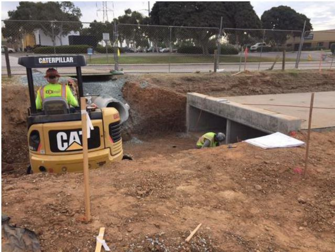
Photo 3: Continuing construction of the box culvert and excavation for the wing walls upstream of the box culvert at the Bay Boulevard Substation southern driveway site was observed this reporting period.
