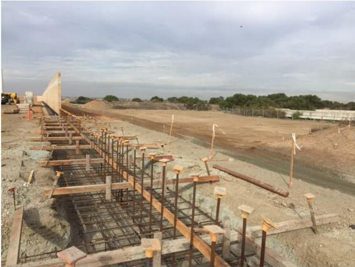
Photo 2: Foundation and masonry work on the construction screening wall (above) and control shelter continued this reporting period.
