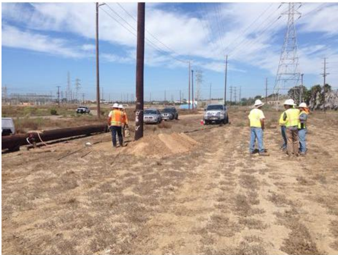
Photo 4: During pole removal and installation along the transmission alignment, biological and archaeological monitors were observed on site in accordance with APM-BIO-01, APM-BIO-02, and MM-CUL-01, and APM-CUL-05. Paleontological monitors were observed in areas potentially affecting the Bay Point Formation in accordance with APM-CUL-5.
