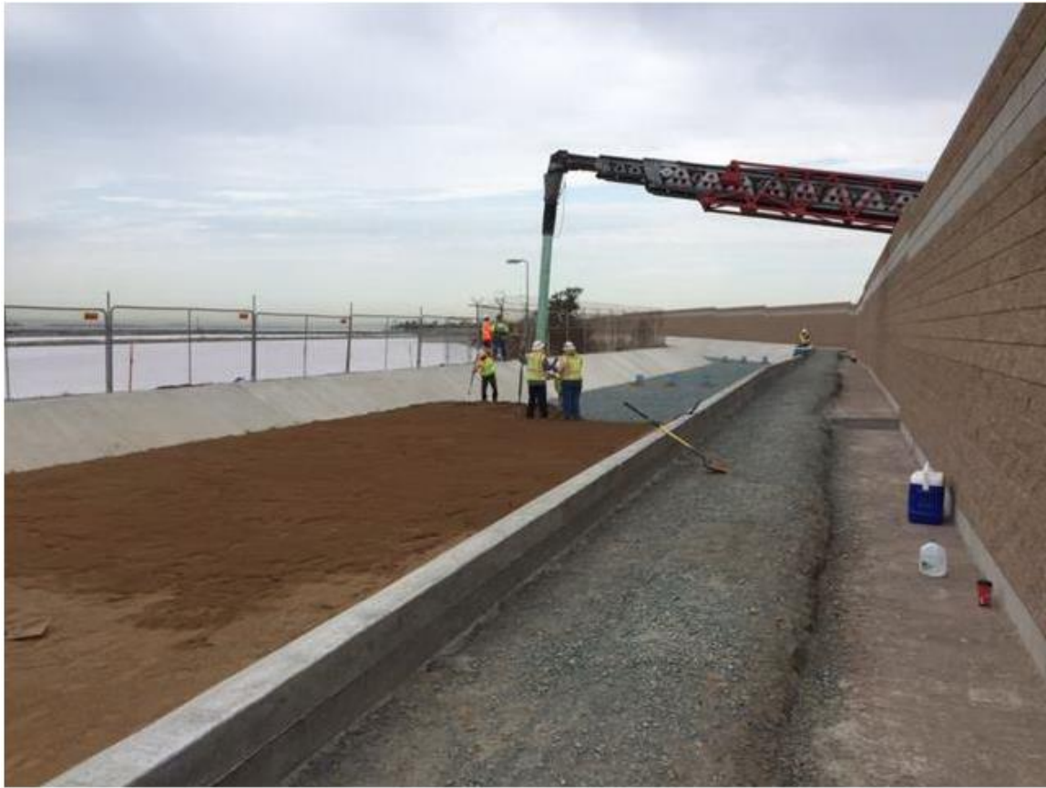
Photo 1: Construction crews were observed placing engineered fill in the bioretention basin during this reporting period.
