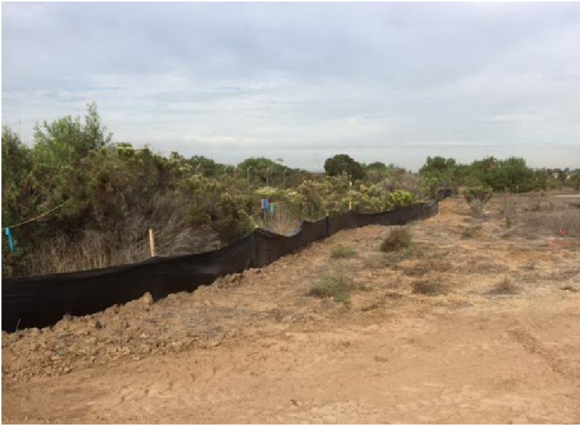
Photo 5: Silt fencing and “Environmentally Sensitive Area” signs were used to protect jurisdictional features along the transmission line alignment.
