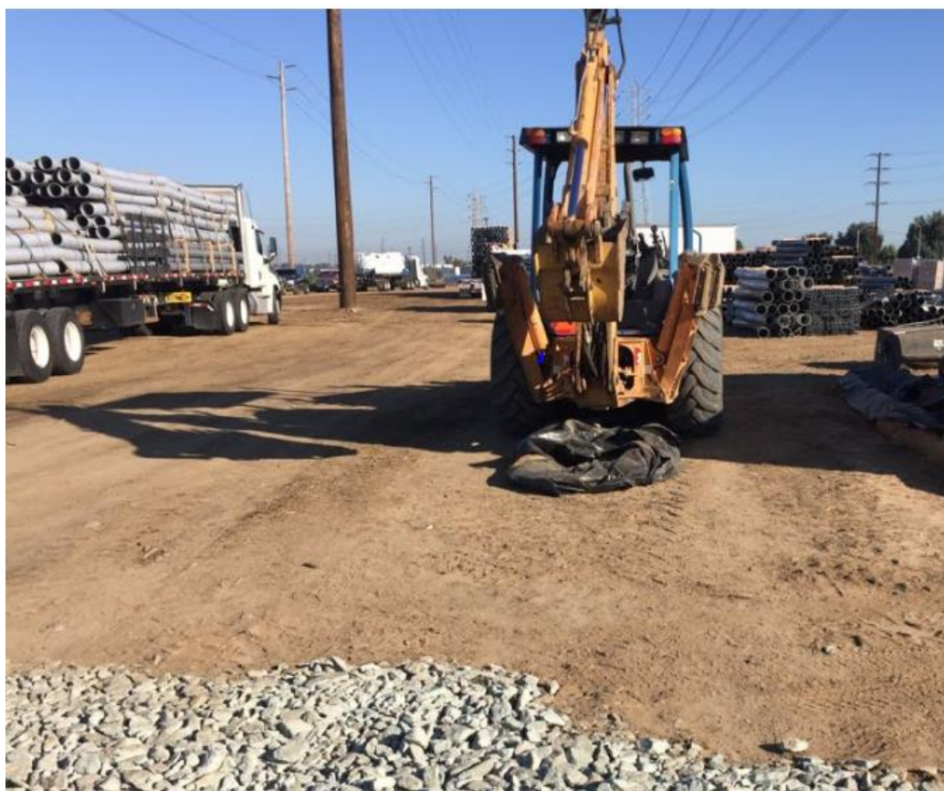
Photo 6: Equipment including dumpsters, heavy vehicular equipment, building materials, etc. was staged along the transmission line alignment. Silt fencing was installed around staging areas, waste bins were observed contained, absorbent material was observed under staged vehicular equipment (above), and dumpsters were observed covered and secured to prevent attracting wildlife.
