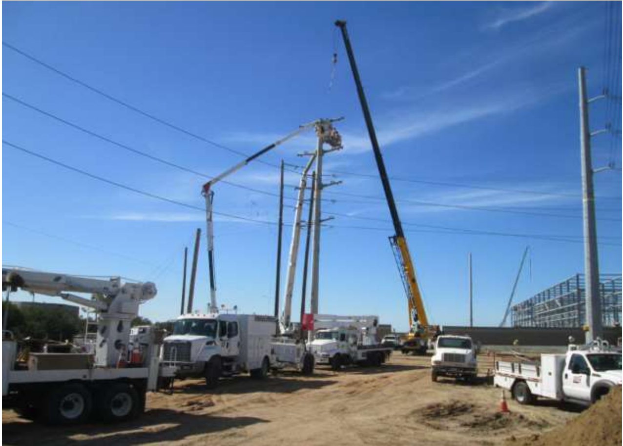
Photo 2: Crews were observed installing a riser pole outside the Bay Boulevard Substation. The riser pole is being installed to tie-in existing circuits into the Bay Boulevard Substation.
