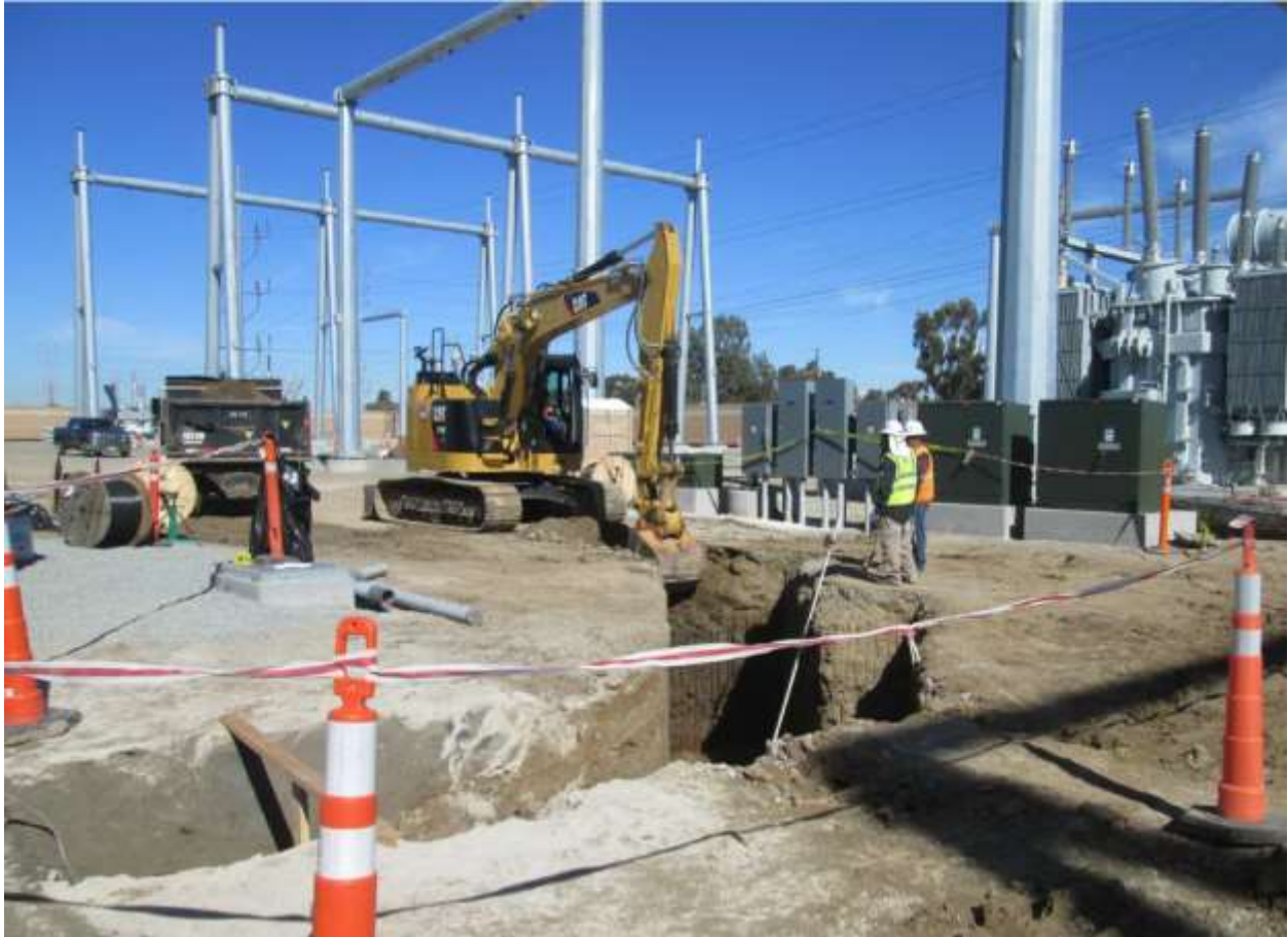
Photo 1: Crews were observed excavating areas within Bay Boulevard Substation to support underground duct banks.
