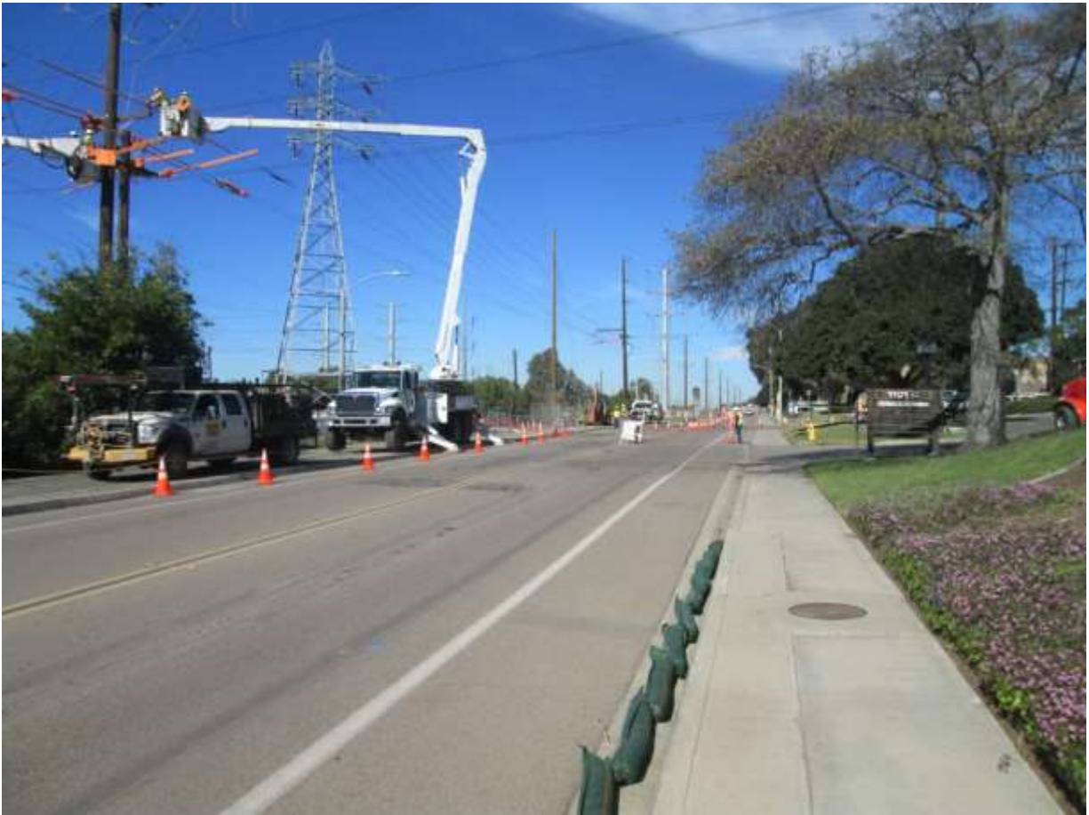
Photo 3: Crews were observed switching out 69kV poles along Bay Boulevard. Traffic control flaggers and signs were used to direct traffic around work areas in accordance with the Traffic Control Plan (MM TRA-01). Gravel bags were installed for inlet protection (right) in accordance with the SWPPP (MM HYDRO-1).
