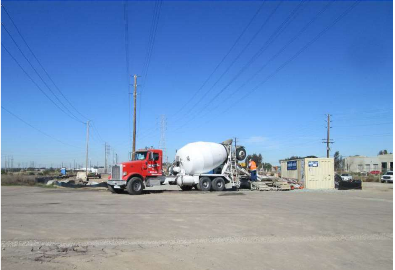
Photo 4: Crews were observed using designated concrete washout stations while working along active areas within the transmission right-of-way corridor per the SWPPP (MM HYDRO-1).
