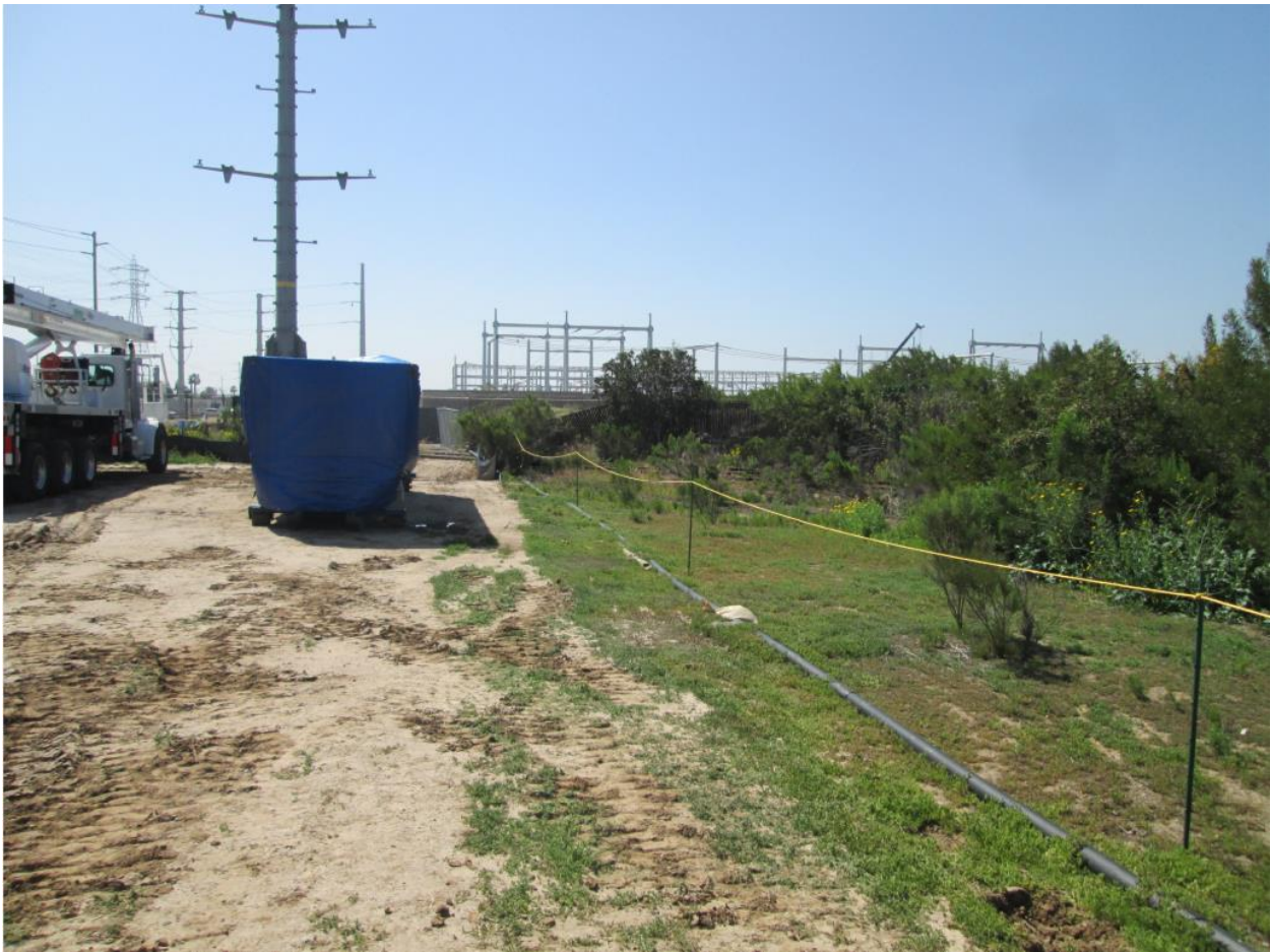
Photo 2: Crews were observed adhering to delineated work limits (as shown above) along the transmission line right-of-way.
