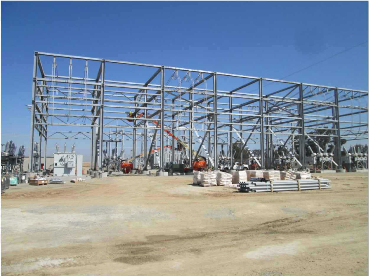
Photo 1: Crews were observed hanging cable within the 69 kilovolt (kV) racks within the Bay Boulevard Substation.
