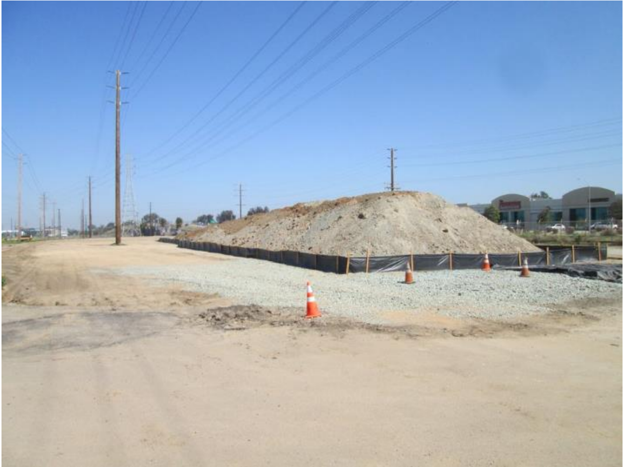
Photo 3: Crews were observed maintaining silt fencing around soil stockpiles along the transmission line right-of-way in accordance with the SWPPP (MM HYDRO-1).
