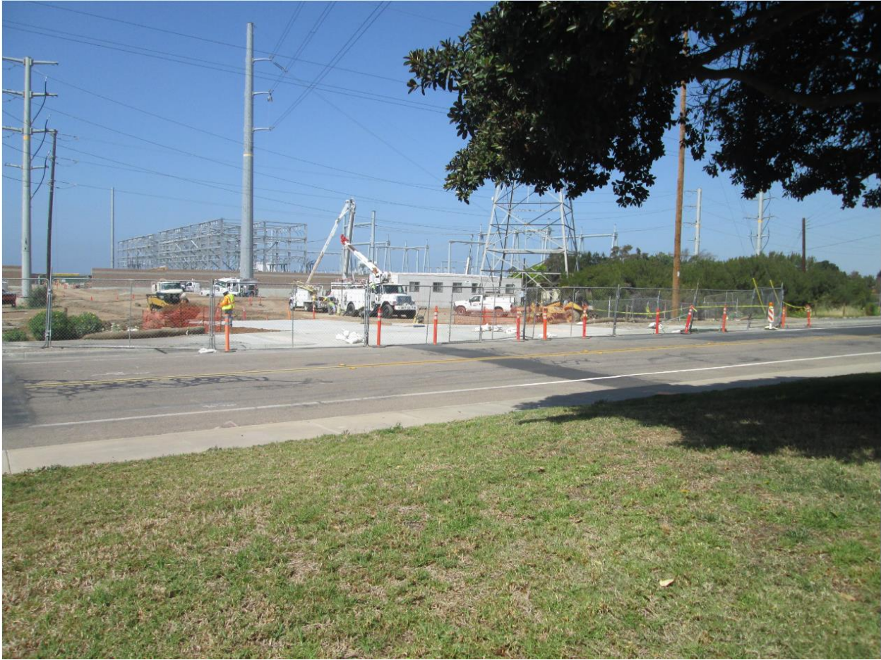
Photo 4: Traffic control signs notifying closure of the adjacent bike path were placed around work areas in accordance with the Traffic Management Plan (MM TRA-01).
