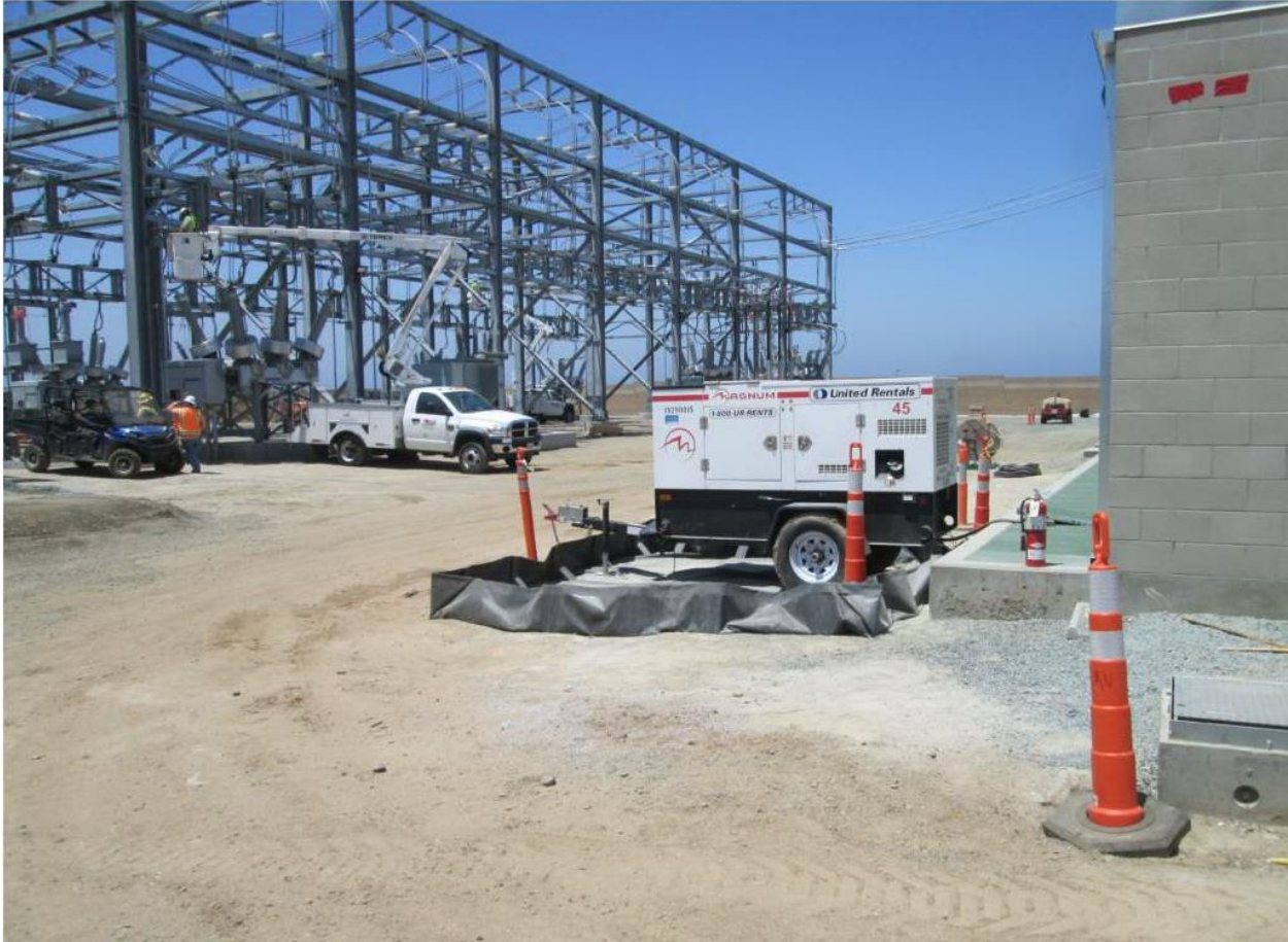
Photo 4: Crews were observed staging vehicular equipment on absorbent padding and within containment in accordance with SWPPP (MM-HYDRO-1) BMPs.
