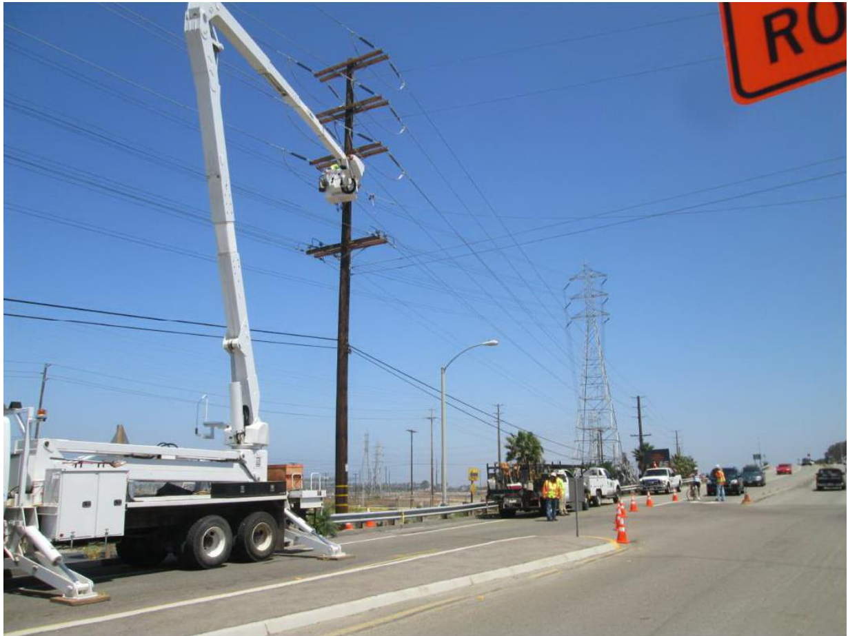
Photo 2: Crews were observed working on a 69kV pole along Bay Boulevard and utilizing traffic control measures (flaggers, cones, and signage) in accordance with the Traffic Management Plan, as required by MM TRA-1. Signs noting short-term closures were also observed along the bike path in accordance with the Traffic Management Plan.
