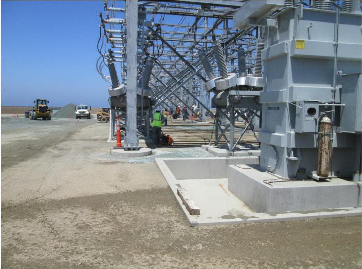
Photo 1: Crews were observed placing Class II base within the Bay Boulevard Substation.
