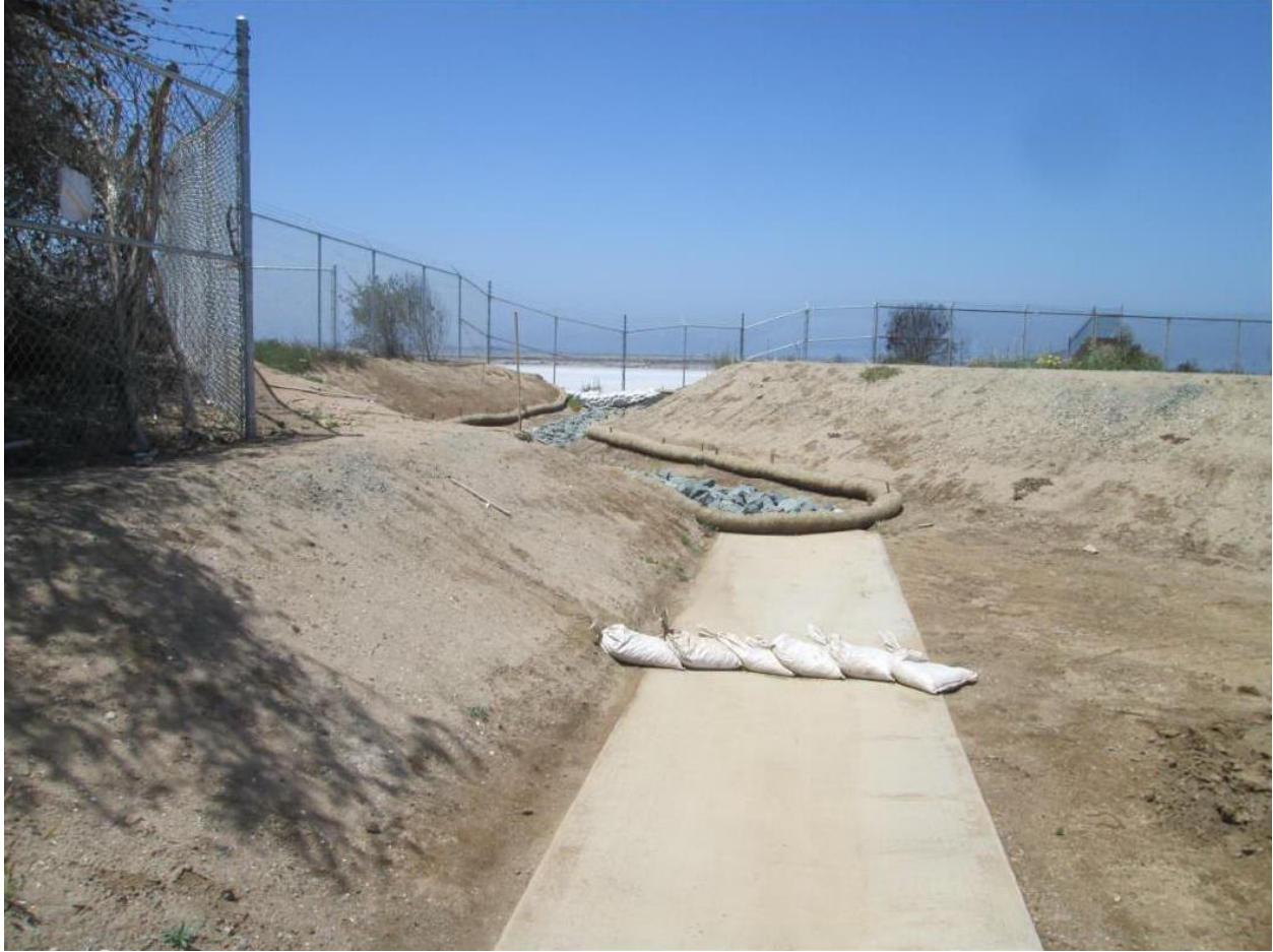
Photo 3: SWPPP (MM HYDRO-1) BMPs (such as fiber rolls and gravel bags, shown above) were observed and drainages were observed free of sediment.
