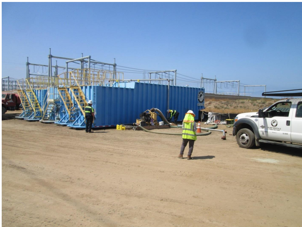
Photo 2: Crews were observed demobilizing frack tanks used to store recycled water on site.
