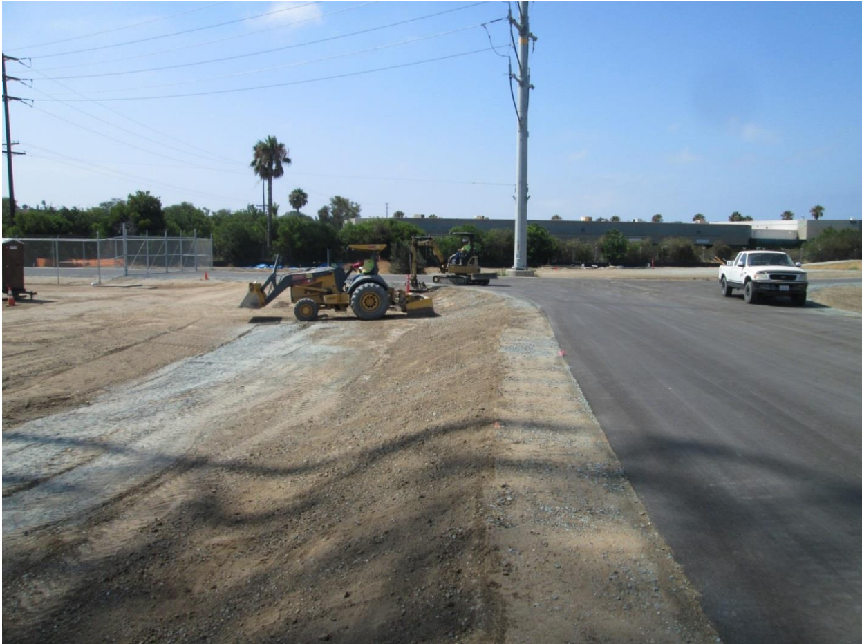
Photo 1: Crews were observed conducting finishing earthwork/grading along banks adjacent to the site access road.
