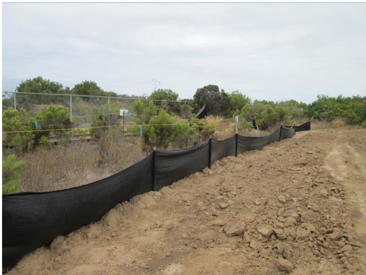
Photo 4: Erosion and sediment control BMPs, such as the use of silt fencing around the flagged environmentally sensitive area, were being maintained in accordance with the project SWPPP (MM-HYDRO-01).
