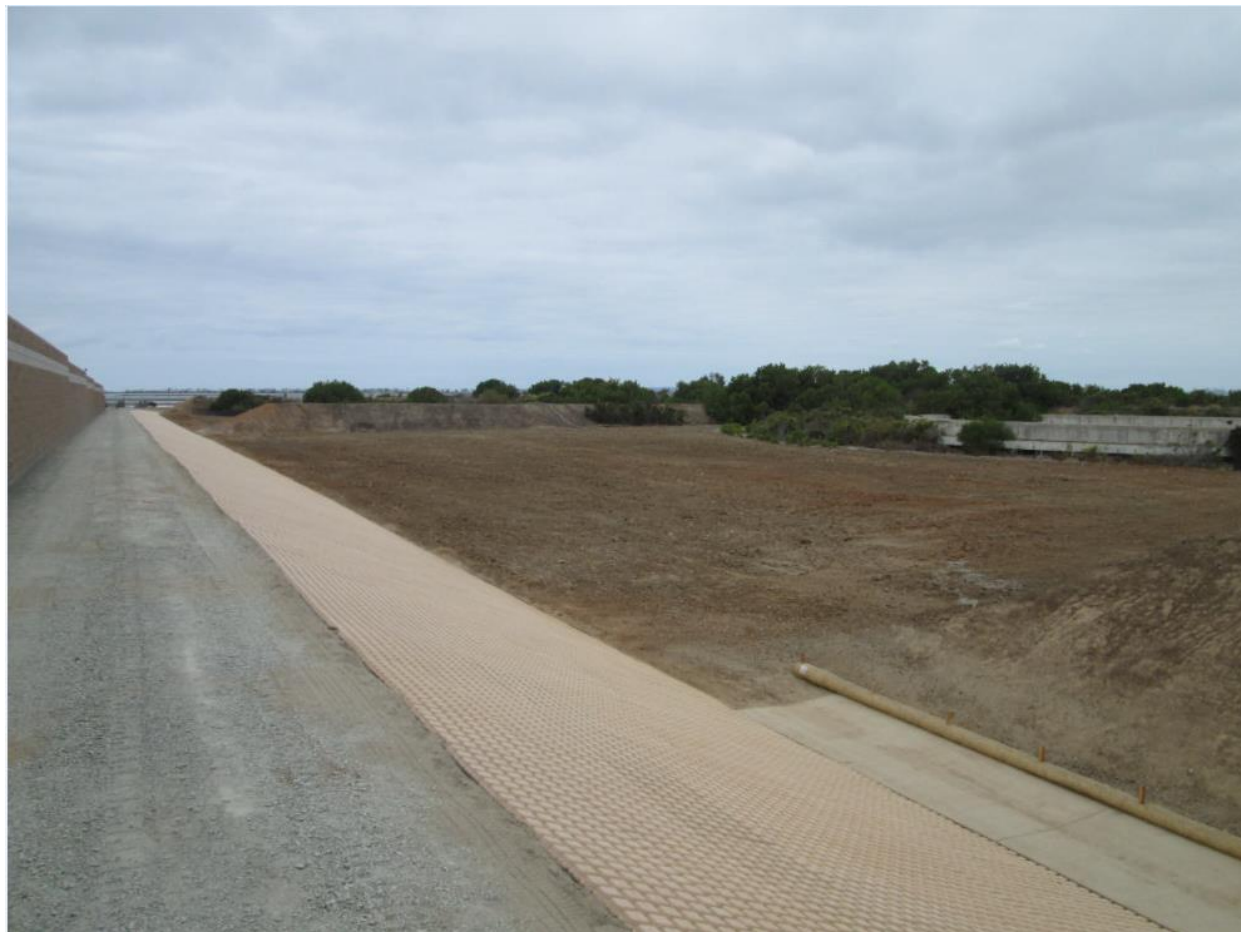
Photo 3: North of the Bay Boulevard Substation, soils within temporary work areas were observed ripped in preparation for final stabilization, permanent pavers were installed along slopes, and SWPPP BMPs including straw wattles (MM-HYDRO-1) were observed installed.
