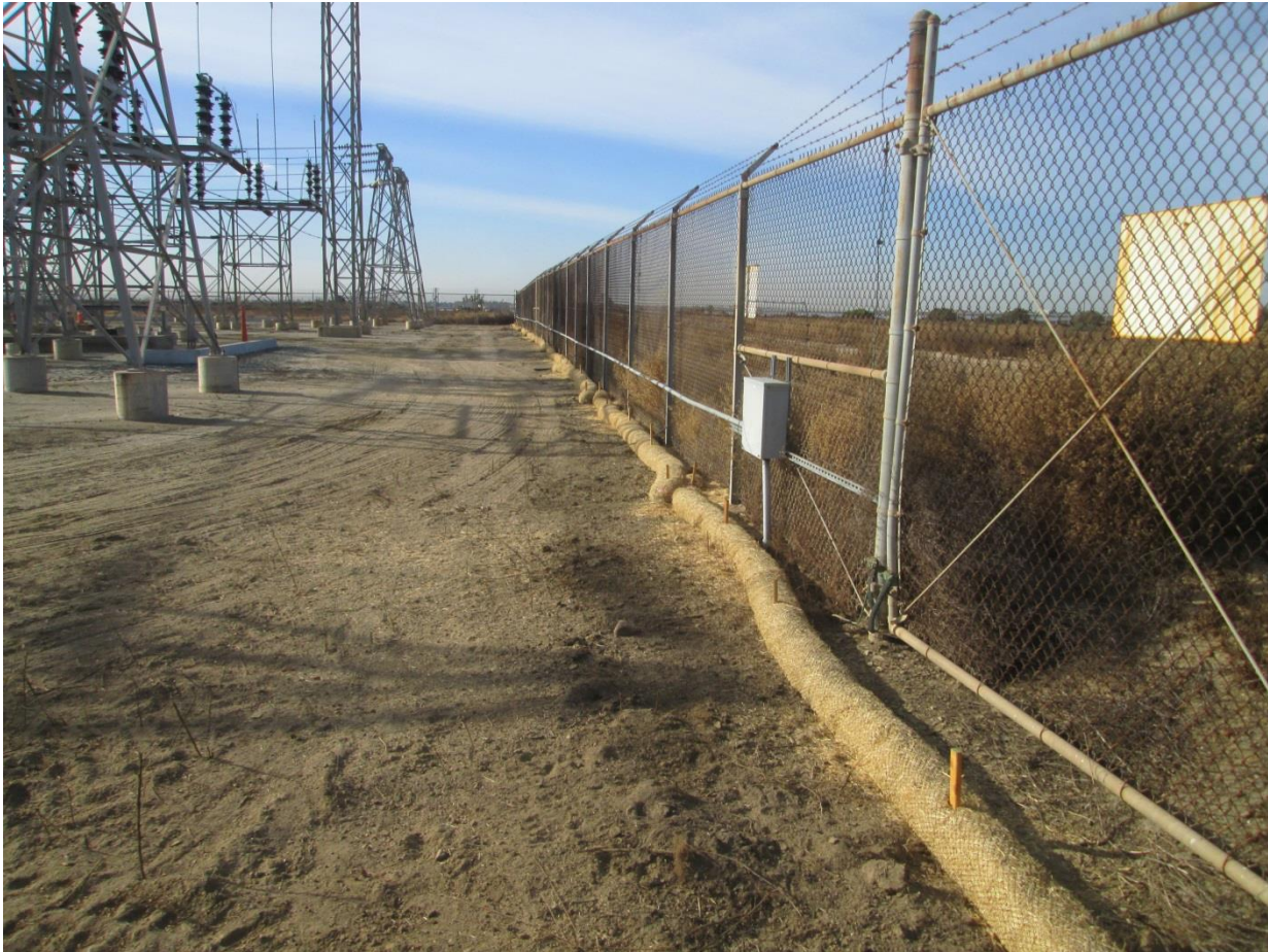
Photo 3: Sediment control BMPs, such as perimeter straw wattles were observed being maintained in accordance with the project SWPPP (MM HYDRO-01).
