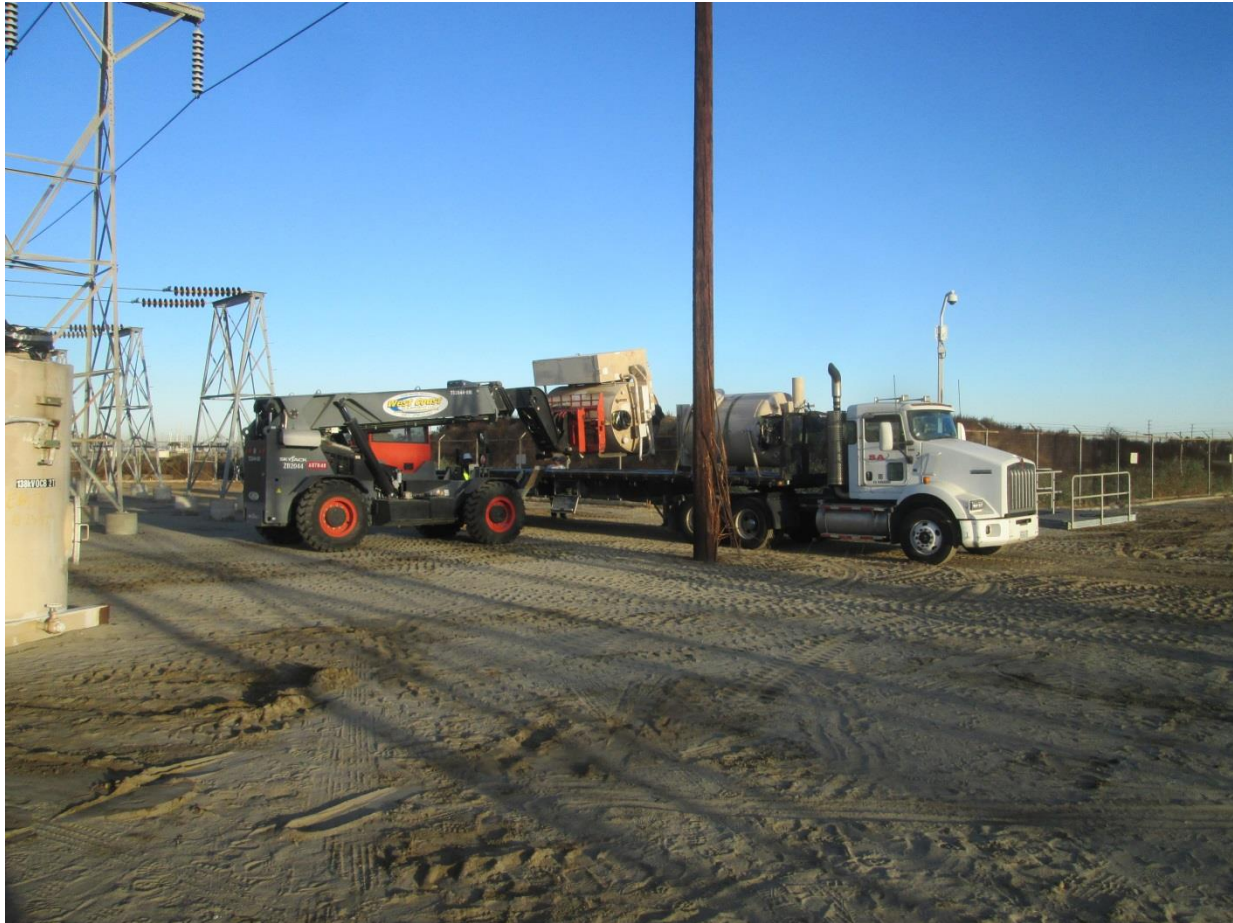
Photo 2: A construction crew observed loading circuit breaker tanks onto a flatbed truck for hauling off site and disposal.
