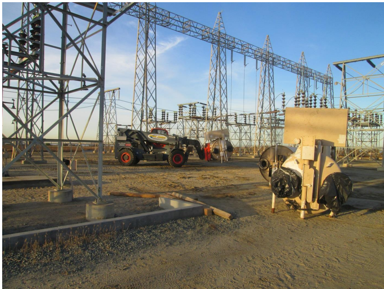
Photo 4: During the removal of circuit breaker tanks, plastic was observed being used to cover openings in the tanks to prevent potential leaks from being discharged into the soil in accordance with the Hazardous Substance Management and Emergency Response Plan (APM HAZ-01).
