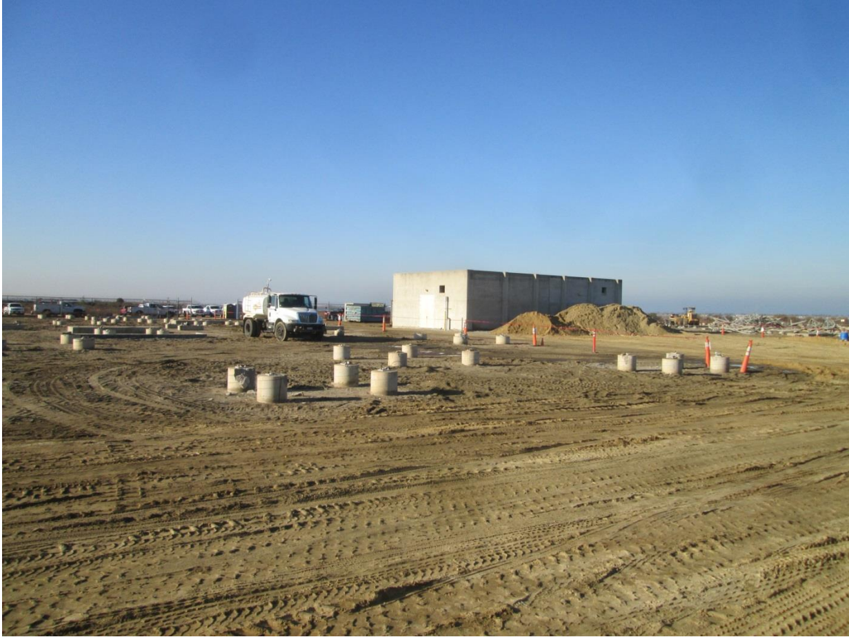
Photo 2: A water truck was utilized for as-needed watering within the work area to prevent dust emissions in accordance with the Dust Control Plan (MM-BIO-5) and APM-AIR-01.
