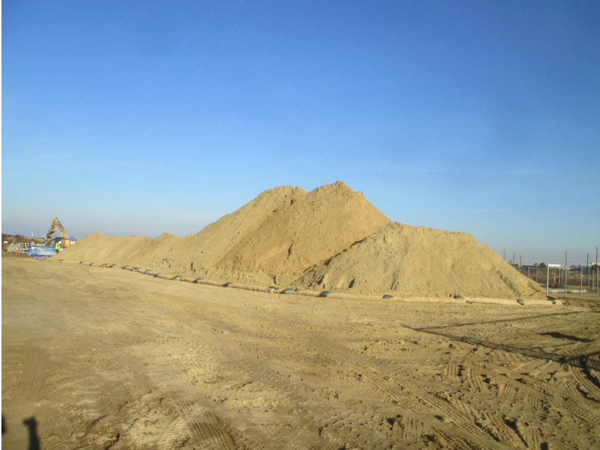
Photo 4: Sediment control devices such as fiber rolls and gravel bags were observed being used for stockpile management around the perimeter of an imported dirt stockpile (to be used for backfill) in accordance with the Storm Water Pollution Prevention Plan (MM-HYDRO-1).
