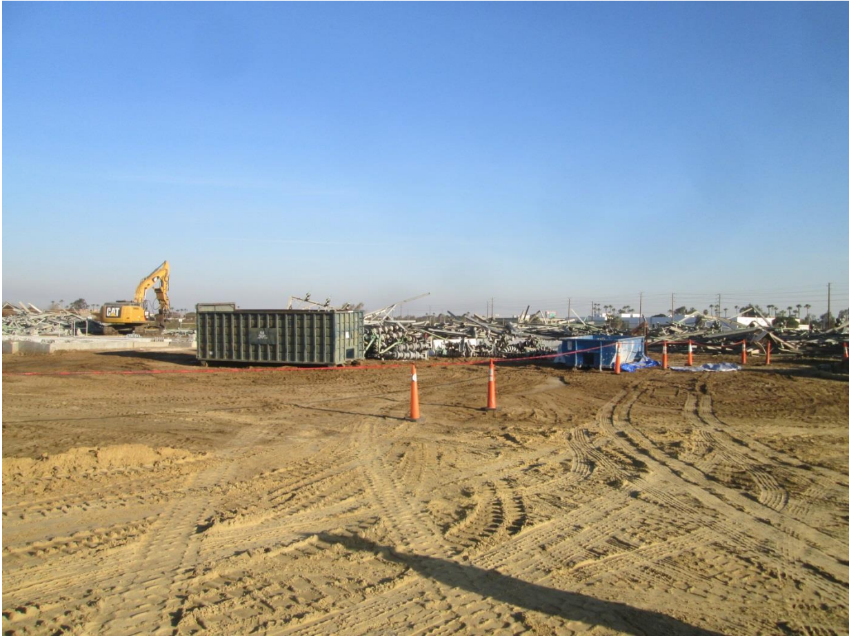
Photo 1: A construction crew observed using a shear to cut and stockpile structural steel scrap at the South Bay Substation demolition site in preparation for hauling to an off-site recycling facility.
