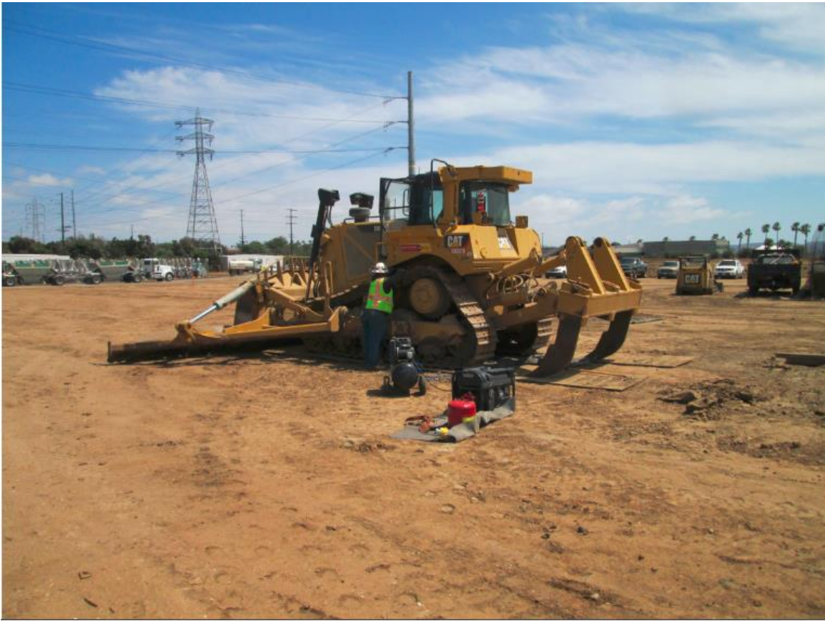
Photo 6: Crews were observed cleaning mud from equipment prior to hauling offsite to prevent sediment track-out from the project in accordance with the project SWPPP and to reduce potential for offsite transport of weedy material in accordance with MM BIO-04.
