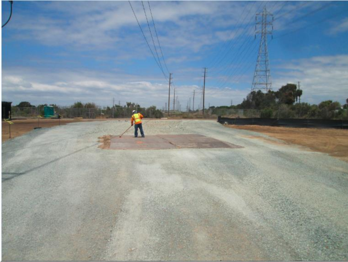
Photo 5: Crews were observed maintaining sediment track-out BMPs (sweeping rattle plates) throughout the project site in accordance with the project SWPPP (MM HYDRO-01).
