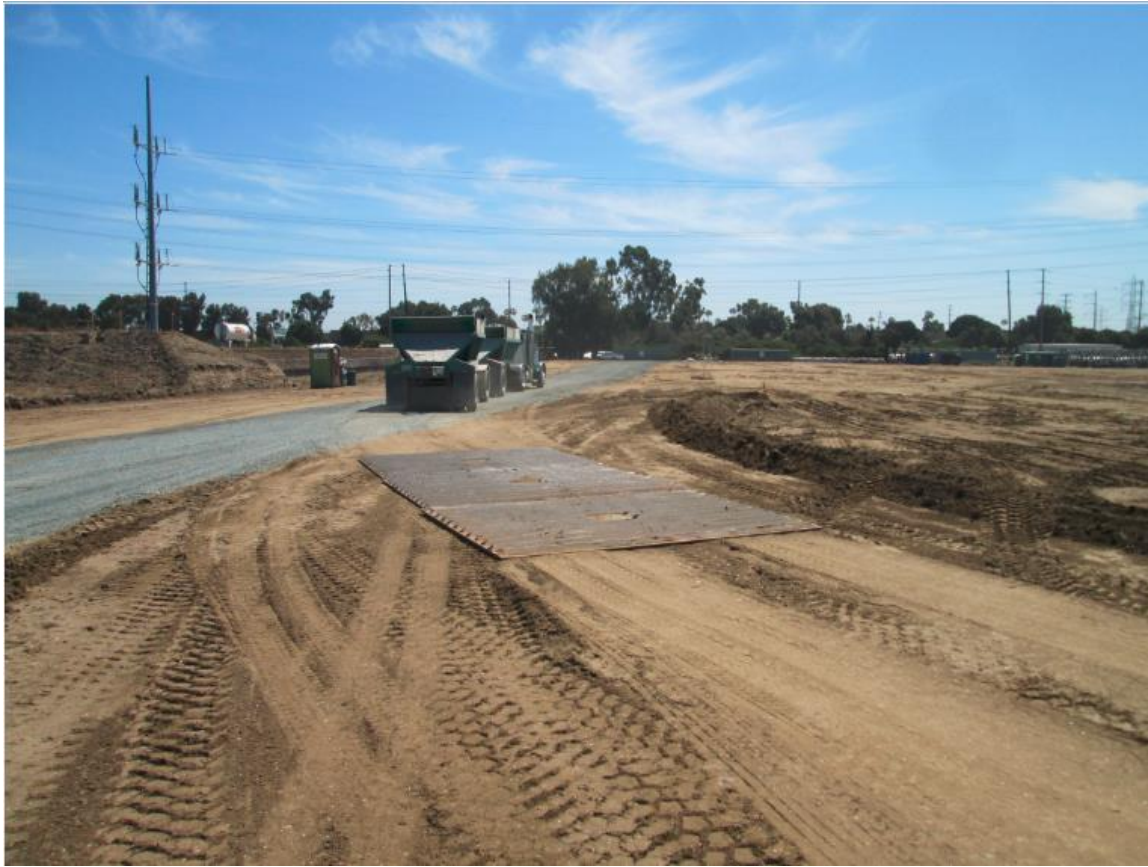
Photo 4: Within the project site, a haul road for trucks carrying imported fill material was created, with additional Class II base added to prevent potential of sediment track out from the project site. Additional rattle plates were installed at the intersection of the haul road and the grading/excavation/compaction areas to further prevent off-site sediment track out in accordance with the project SWPPP.
