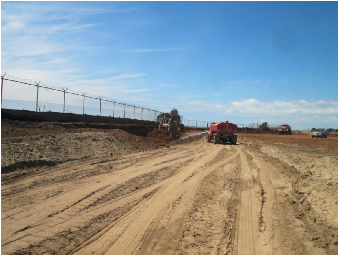
Photo 2: Water trucks carrying reclaimed water were used to prevent dust emissions on site during excavation activities (water retention basin, above) in accordance with APM AIR-01.
