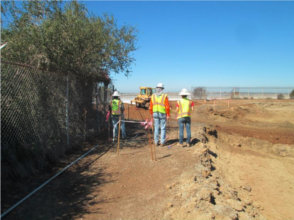
Photo 1: Archaeological and paleontological monitors observing excavation and re-compaction activities in accordance with MM CUL-01 and APM CUL-05.
