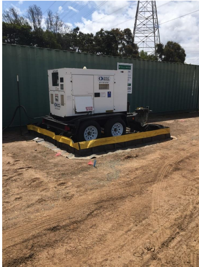
Photo 3: Spill prevention measures included secondary containment bins under equipment in accordance with APM HAZ-01.
