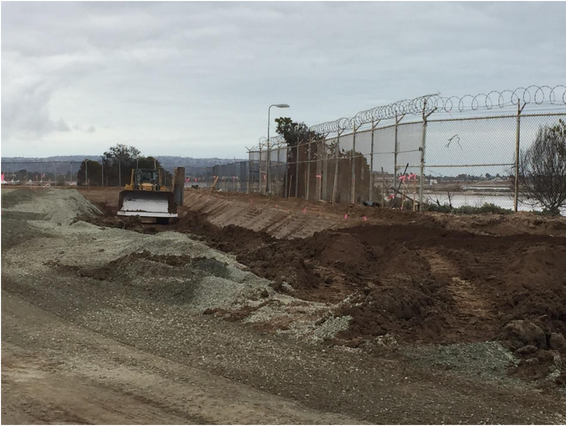
Photo 2: Crews were observed excavating material for the water retention basin along the western internal perimeter of the Bay Boulevard Substation site.
