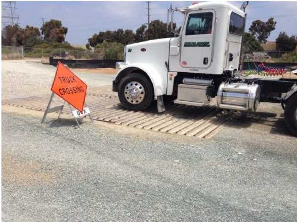
Photo 3: Rattle plates installed at the project entrance, used to minimize sediment track out were observed in good working condition in accordance with the SWPPP. Traffic control signage was observed at the project entrance and along Bay Boulevard in accordance with the Traffic Control Plan (MM-TRA-1).
