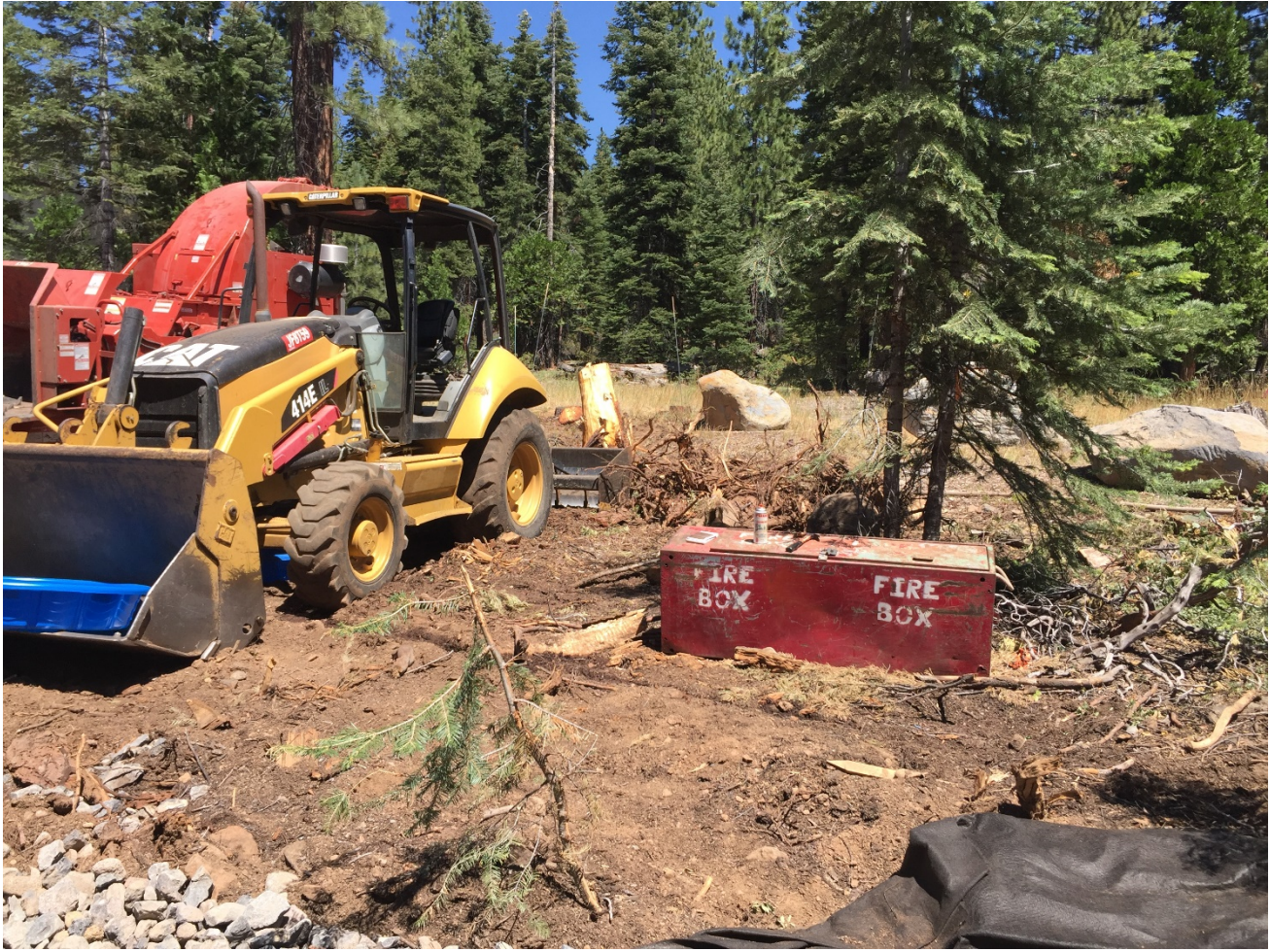
Photo 4: Fire box stored near equipment staging area in accordance with APM-HAZ-6.
