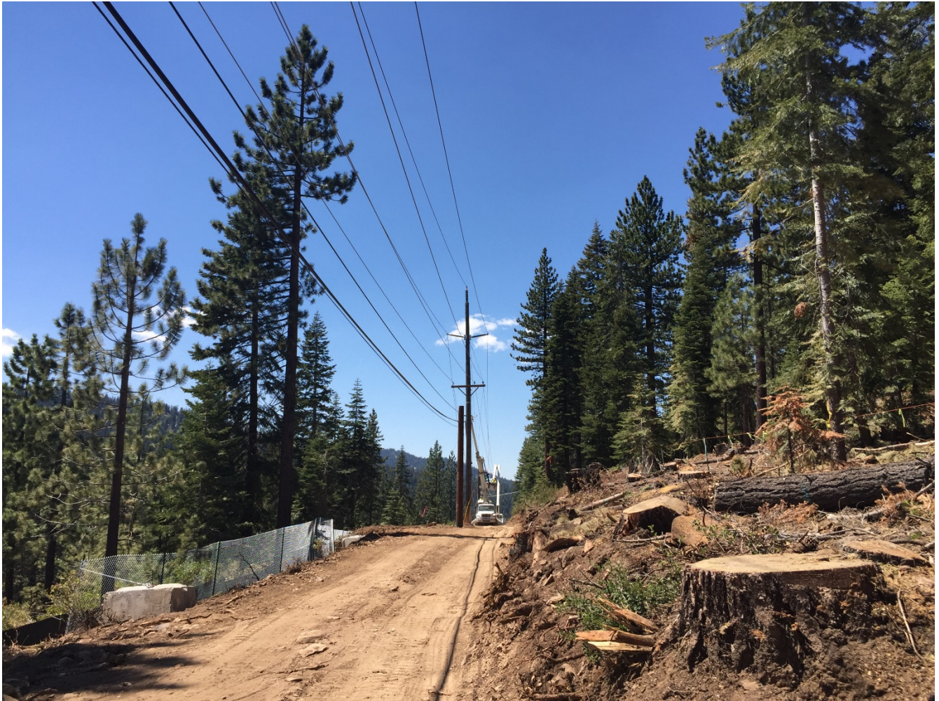
Photo 3: Right-of-way near pole 291156, with debris fence on downhill side to prevent debris rolling down to Highway 267 below. Approved work area roped and flagged along both sides.
