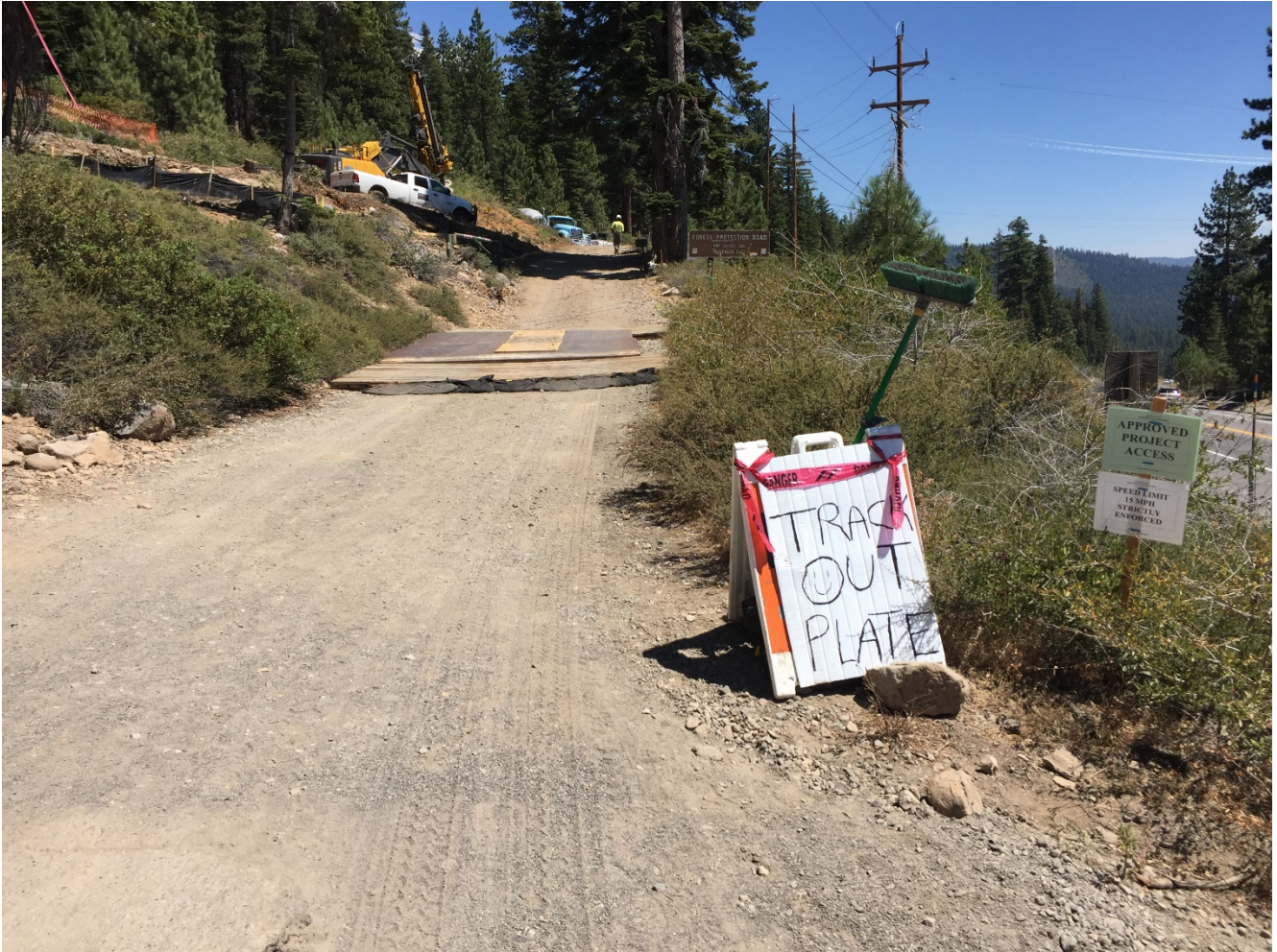
Photo 6: Project access road near Pole 291183, including signage and track-out plates to prevent track-out onto adjacent Highway 267, in compliance with APM-AQ-8.
