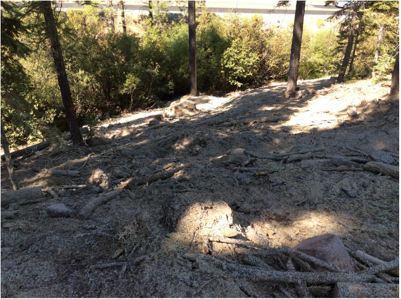
Photo 1: Access road to Pole 291108 covered under Minor Project Refinement #2 regraded, slash scattered, and hydroseed applied.
