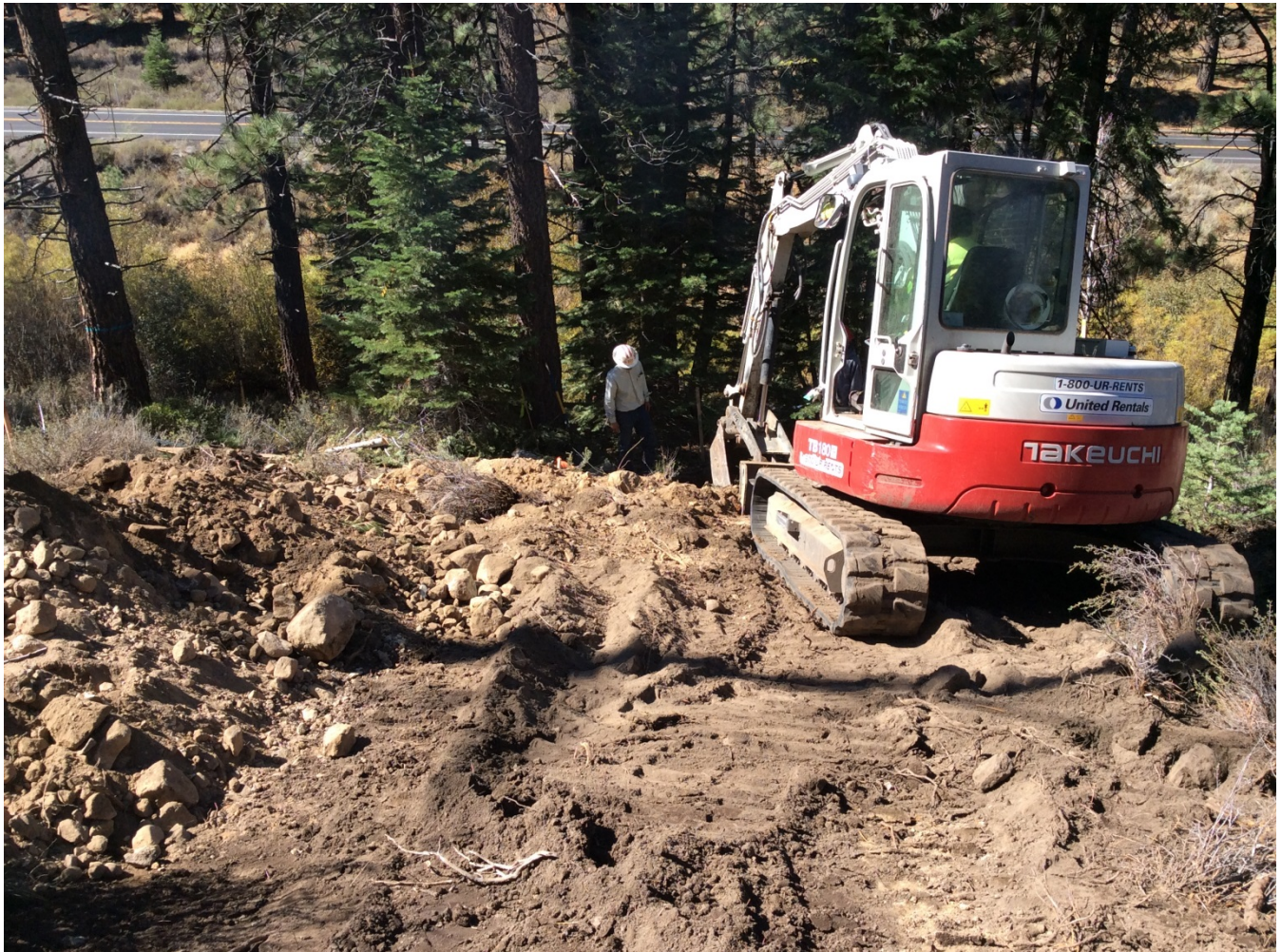
Photo 5: Excavation for pole anchors at Pole #291087 in temporary work areas outside of ROW, as approved under Minor Project Refinement 001. Biological monitor was on-site during excavation activities.
