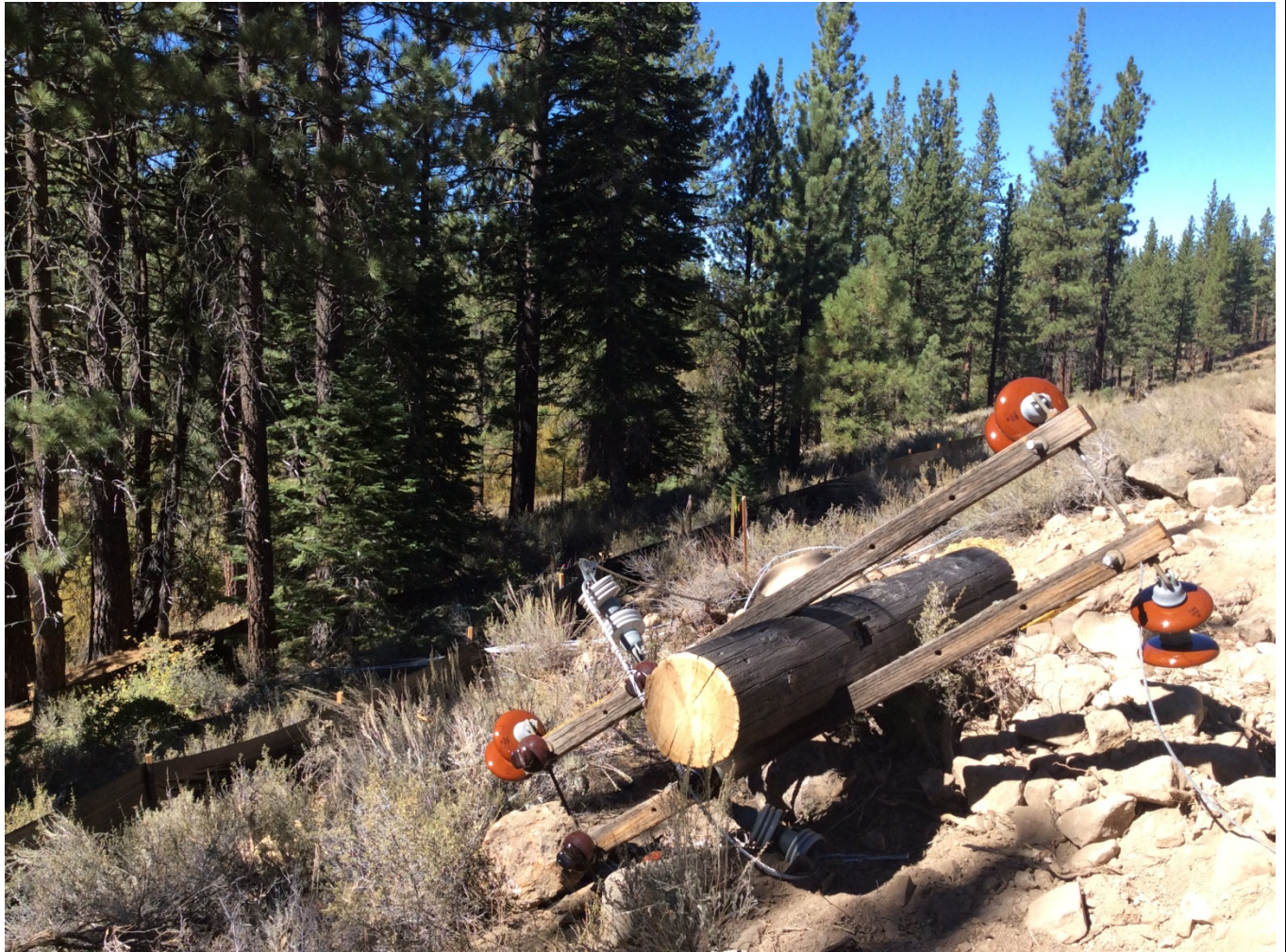
Photo 3: Pole top removed and staged within the ROW to be dismantled and removed from site, near Pole #291087.
