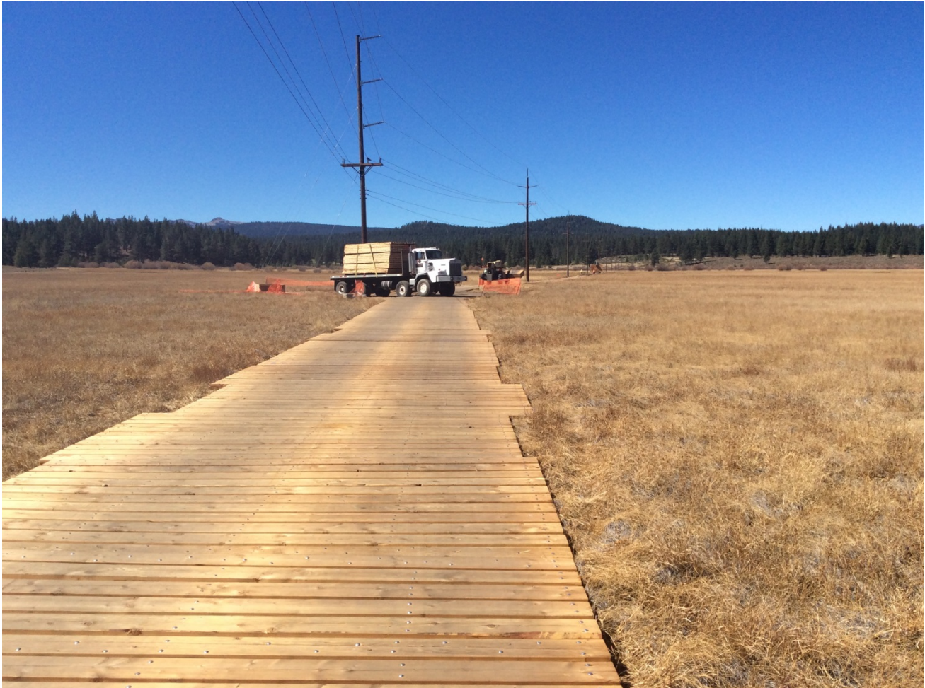
Photo 1: Timber matting being removed in Martis Valley, biological monitors present during removal activities.
