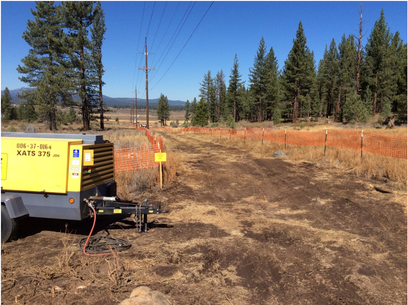
Photo 4: Weed cleaning station with high-pressure air compressor near Pole #291081, in accordance with APM-BIO-6.
