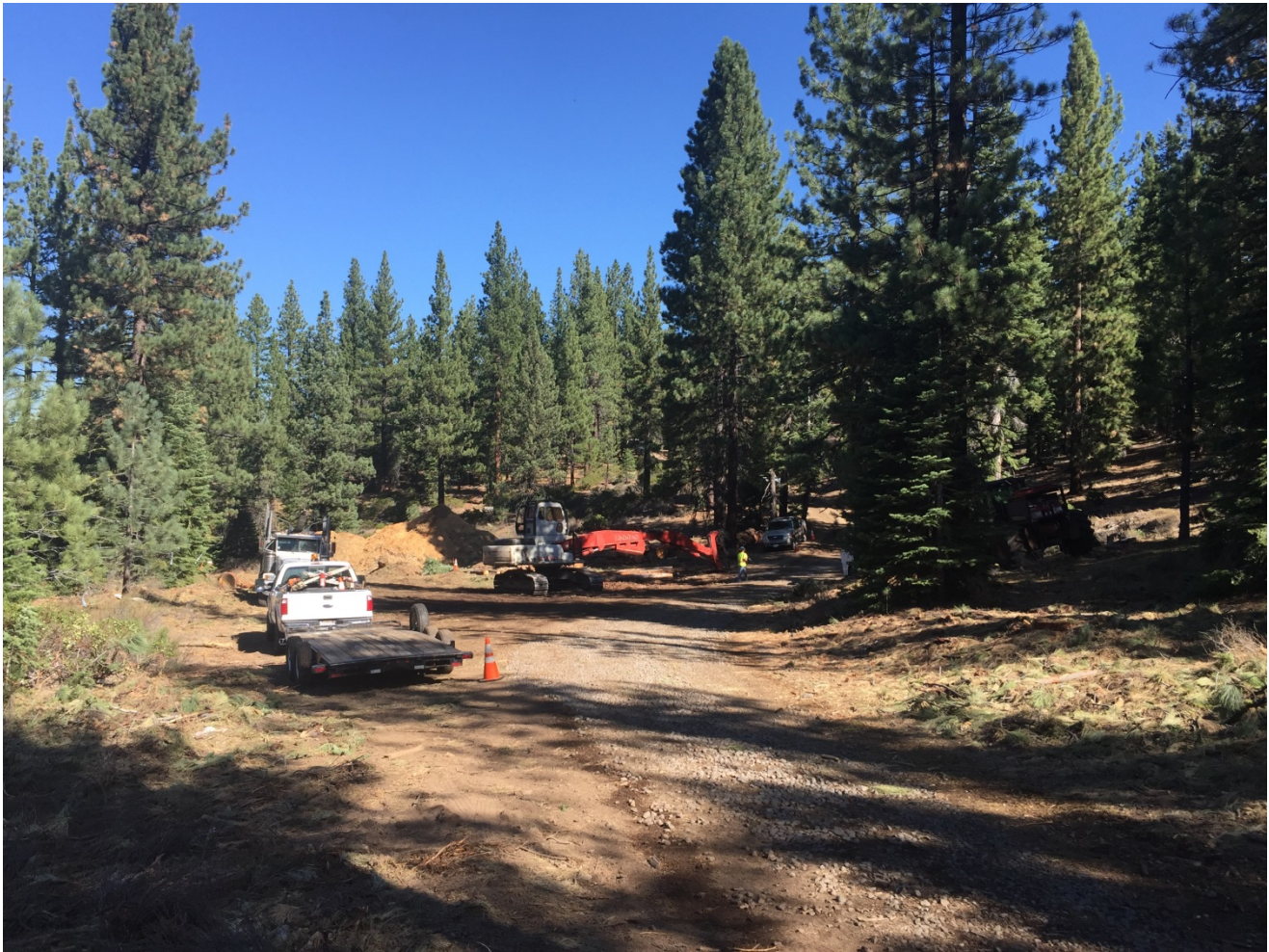
Photo 4: Demobilization at landing for timber operations near Pole #291112. Equipment being removed and erosion control measures being installed.
