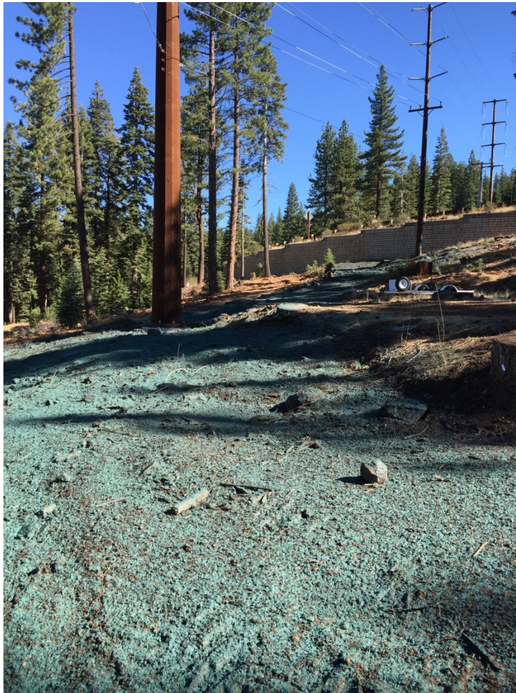
Photo 1: Revegetation/hydroseeding of Northstar fold area along a new ROW alignment, near the Northstar substation.
