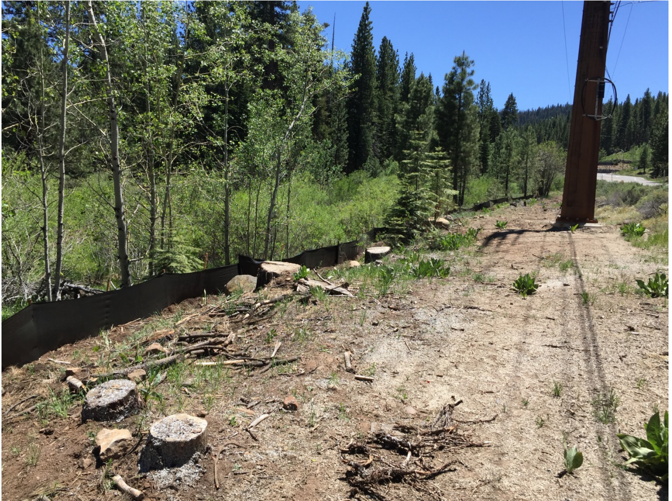
Photo 5: Silt fence being installed along lower edge of ROW prior to construction activities (APM-SOILS-1).
