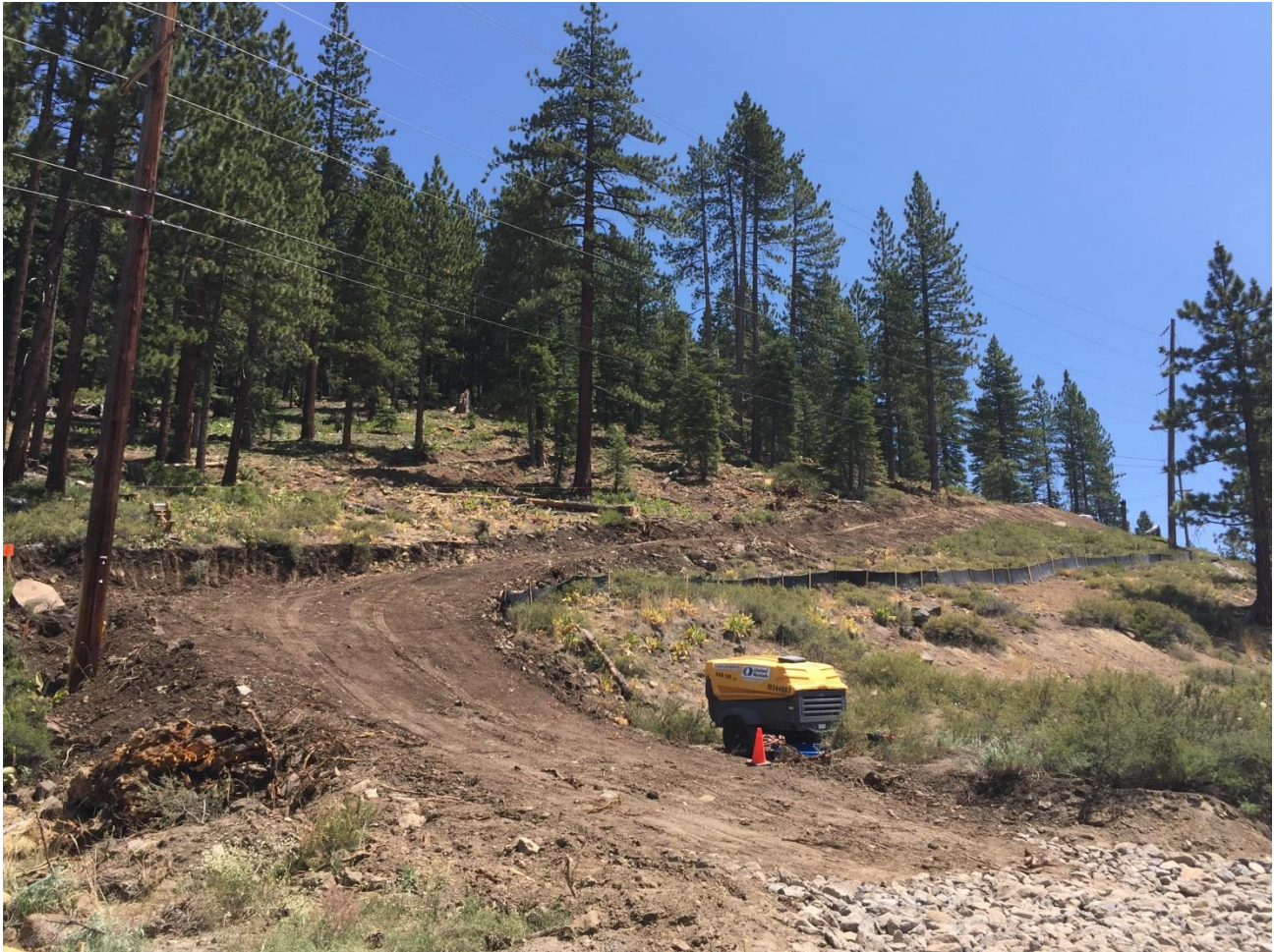
Photo 1: Right-of-way entrance with stabilized rock entrance, weed cleaning station, and silt fence installed below access road.
