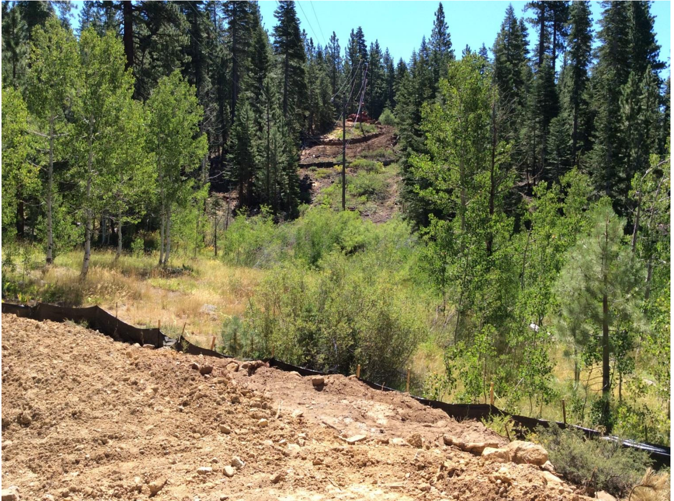
Photo 5: Right-of-way with Pole 291161 in the background. Based on engineering design, the foreground pole(nearest pole) will be removed and not replaced.
