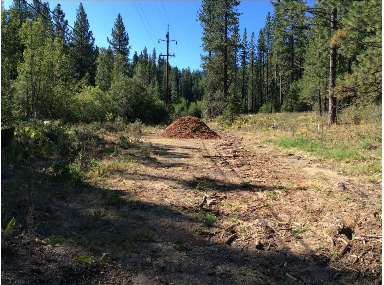
Photo 2: Right-of-way near Pole 291110 following pole installation. Mulch staged for future distribution for erosion control purposes.
