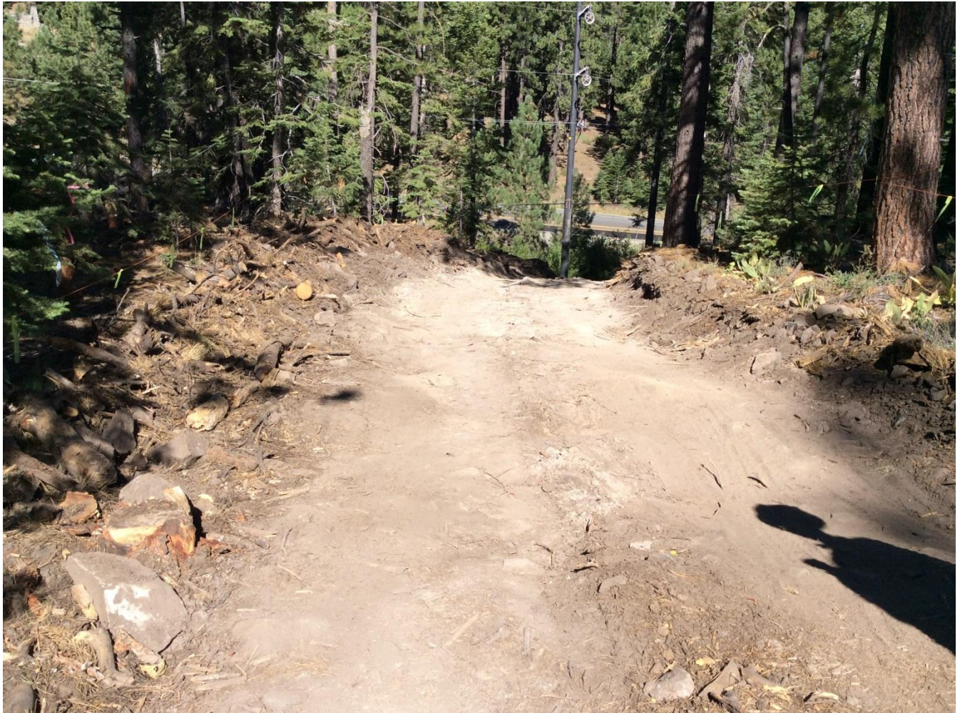
Photo 3: Temporary access road to Pole 291108, approved with Minor Project Refinement #2. Work area boundaries delineated.
