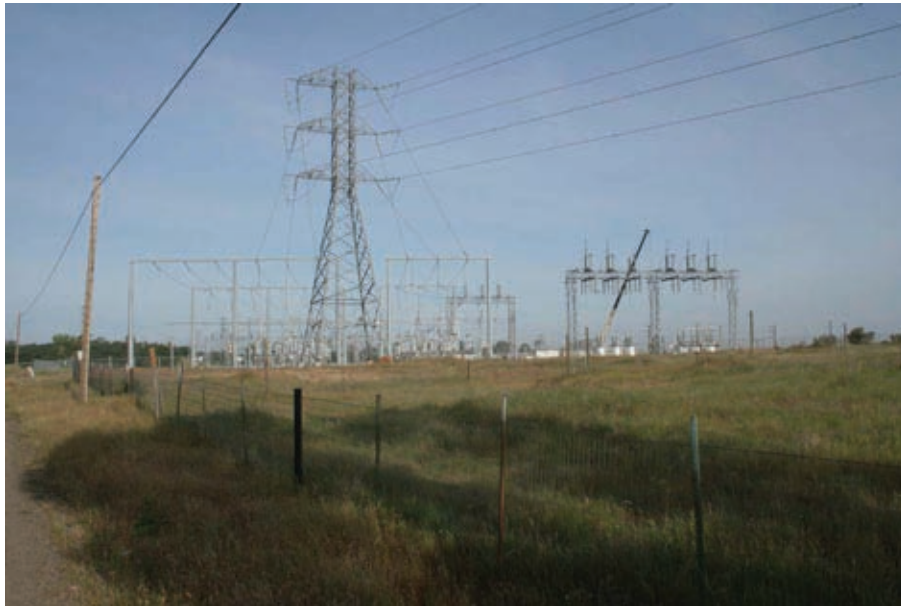
1. Stageline Road looking northwest toward Palermo Substation
