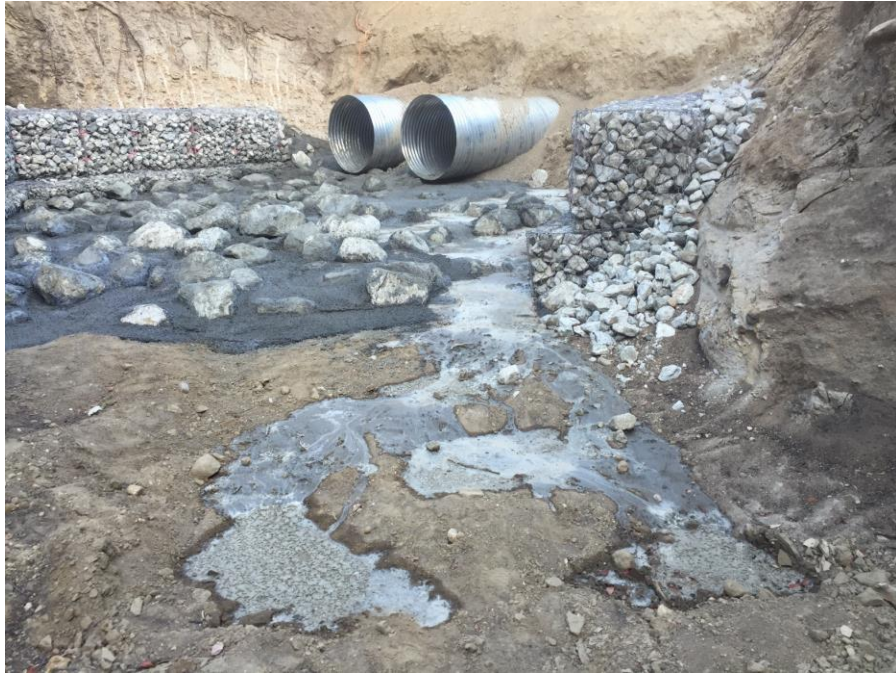
Photo 1: Concrete washout wastewater pooling in Drainage 4. November 4, 2015.
