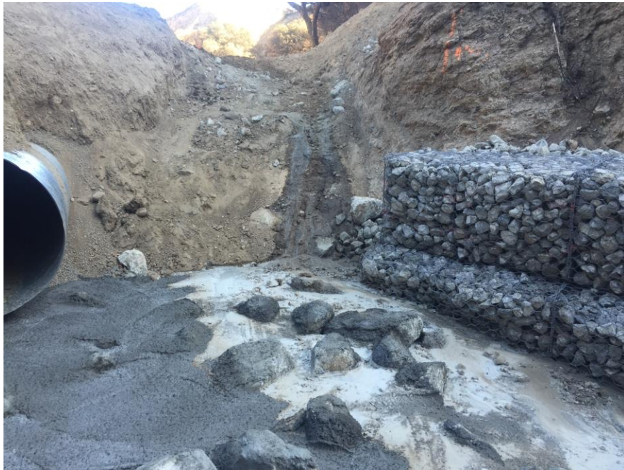
Photo 2: Concrete washout wastewater poured on slope leading to Drainage 4 (lighter color). November 4, 2015.
