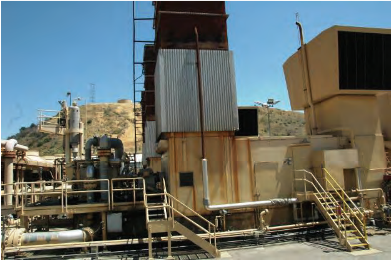
Figure 2 –Complete TDC from left to right: Compressor, gear, exhaust stack, LM1500 housing, air inlet.
