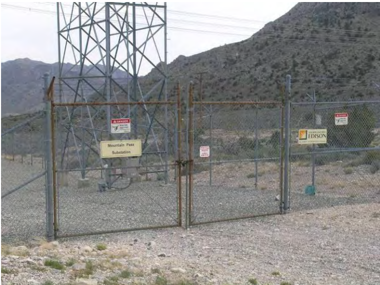
Photograph 15. The existing Mountain Pass Substation. Black bush is dominant here with scattered piñon and juniper.
