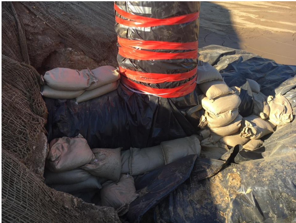
Photo 7: SCE repaired BMPs around the standpipe; plastic sheeting, tape, and additional sandbags reinstalled along the base. Photo taken 1/4/2019, by SCE.
