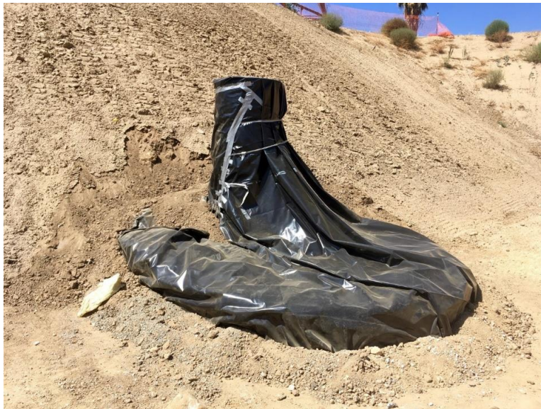
Photo 3: Detention basin standpipe. SCE installed plastic Visqueen sheeting over the standpipe, including the perforations along the base. Photo taken 9/19/2019.
