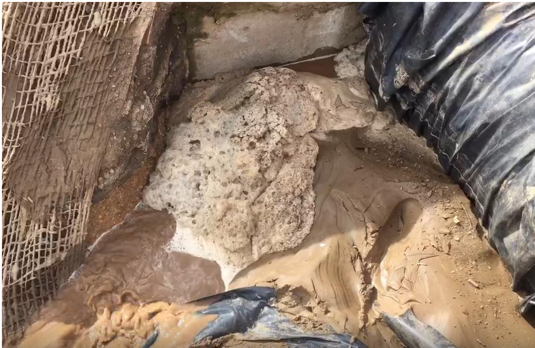
Photo 9: Water rapidly exiting the detention basin from area near the bottom of the standpipe following dewatering of a conduit vault. Water flowing under the plastic sheeting. Photo taken 1/28/2019.
