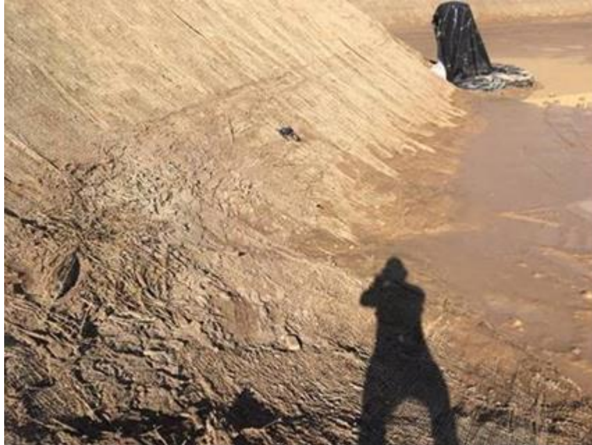
Photo 4: Water line from recent major rain event visible along the banks of the detention basin (water line extends approximately 4-5 feet above the floor of basin). Basin has minimal standing water remaining despite recent high water levels. Photo taken 12/11/18.
