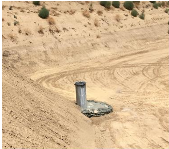
Photo 2: Detention basin standpipe with added gravel and gravel bags at base. Photo taken 8/28/2018.
