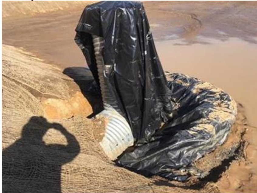
Photo 5: Failed plastic Visqueen sheeting and sandbags surrounding the basin. Perforations visible at base of standpipe. Photo taken 12/11/18.
