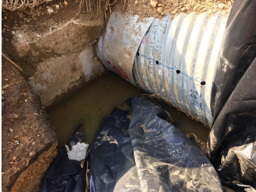
Photo 6: Close-up of the standpipe in the detention basin, with perforated holes allowing sediment-polluted water to quickly run offsite. Photo taken 12/11/2018.
