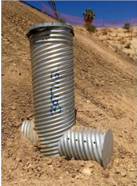
Photo 1: Standpipe in the bottom of the detention basin. Note the perforations along the bottom of the pipe. Photo taken 7/13/2018.
