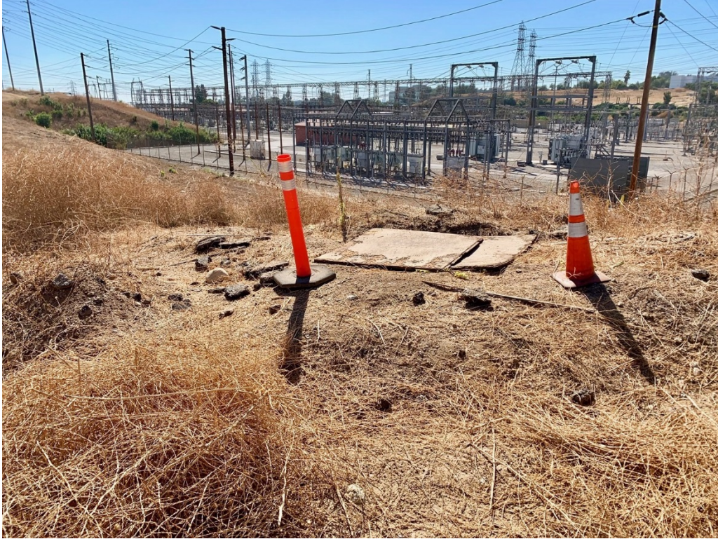
Photo 1. Damaged Manhole M9301070 looking toward the existing substation.
